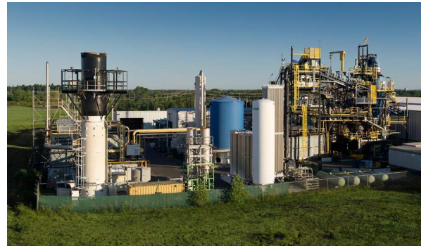
Gasification Pilot Project (Plasco) Ottawa
