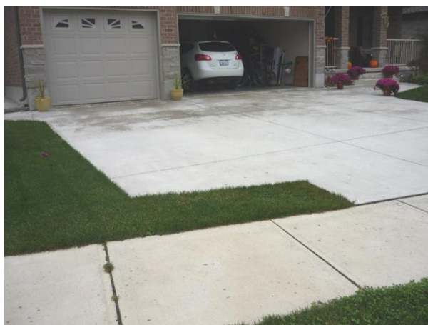
Forced Cut-back of a driveway at street line
