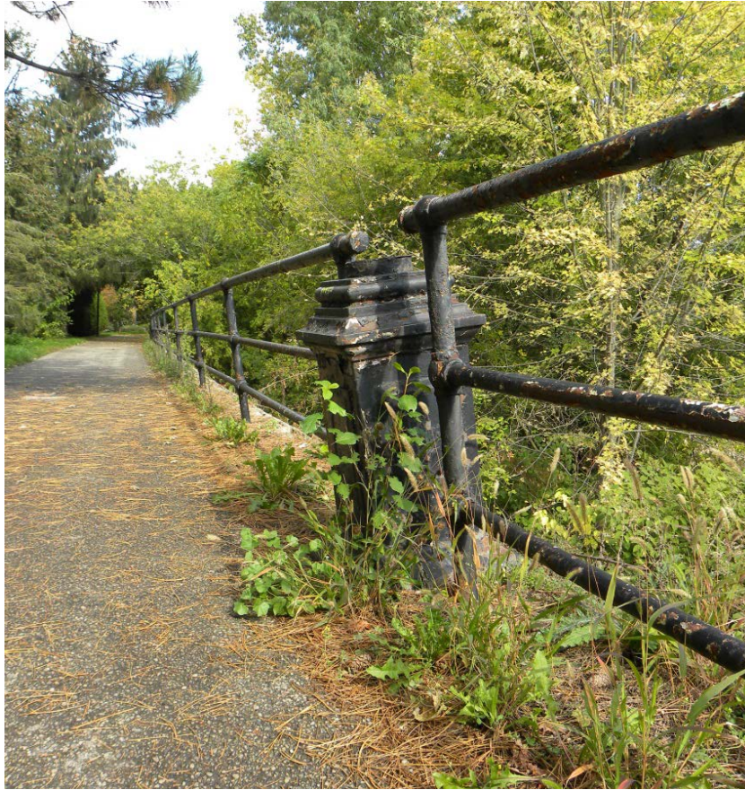
Figure 27: Original hardscape features should be maintained throughout the open spaces in the district.
