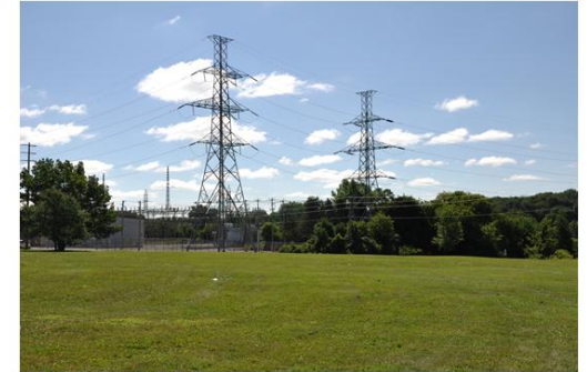
Electrical infrastructure serving the city of London
