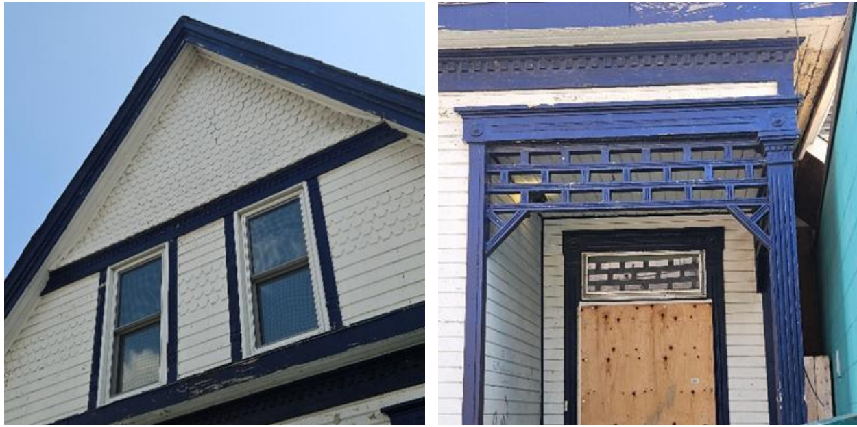
Figures 14-15 – Hexagonal shingles and gable treatment (left) and recessed entrance with fretwork (right)
