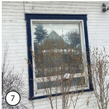
7 Simple window trim with narrow projecting stool/sill and fluted lintel with cornice
