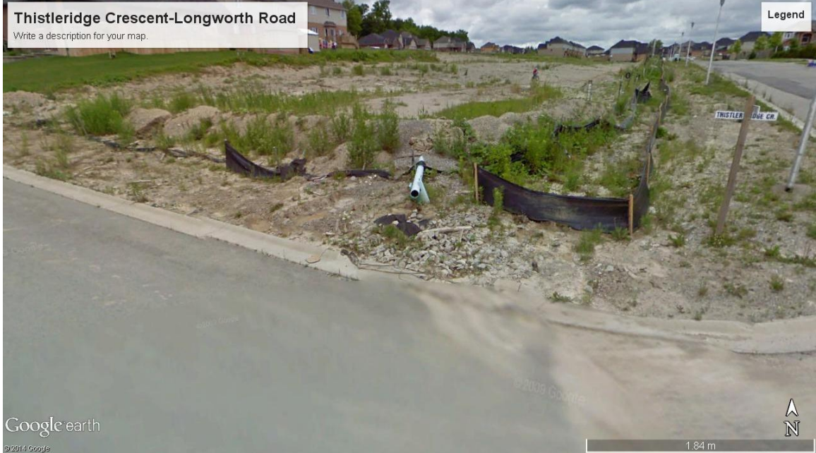
Figure 2. Longworth Road Thistleridge Cresc July 2009. Poor erosion and runoff control. Note: collapsed silt fence, breached berm and scour and sediment export from site (and into PSW).
