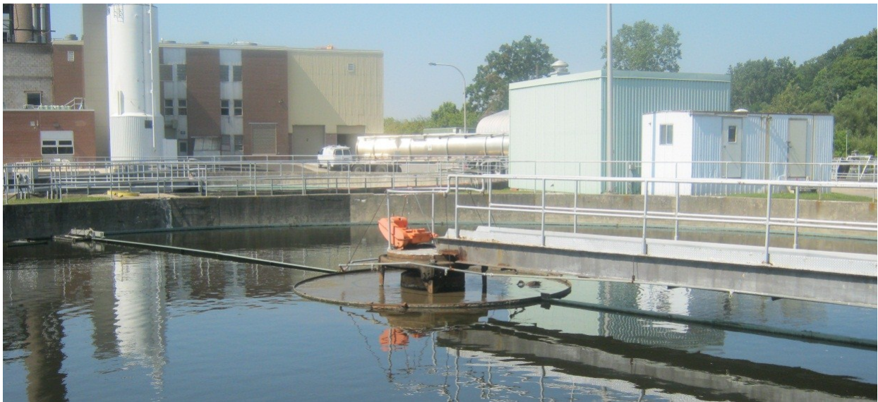
Picture 20 Greenway WWTP Section 1 Final Clarification 2
