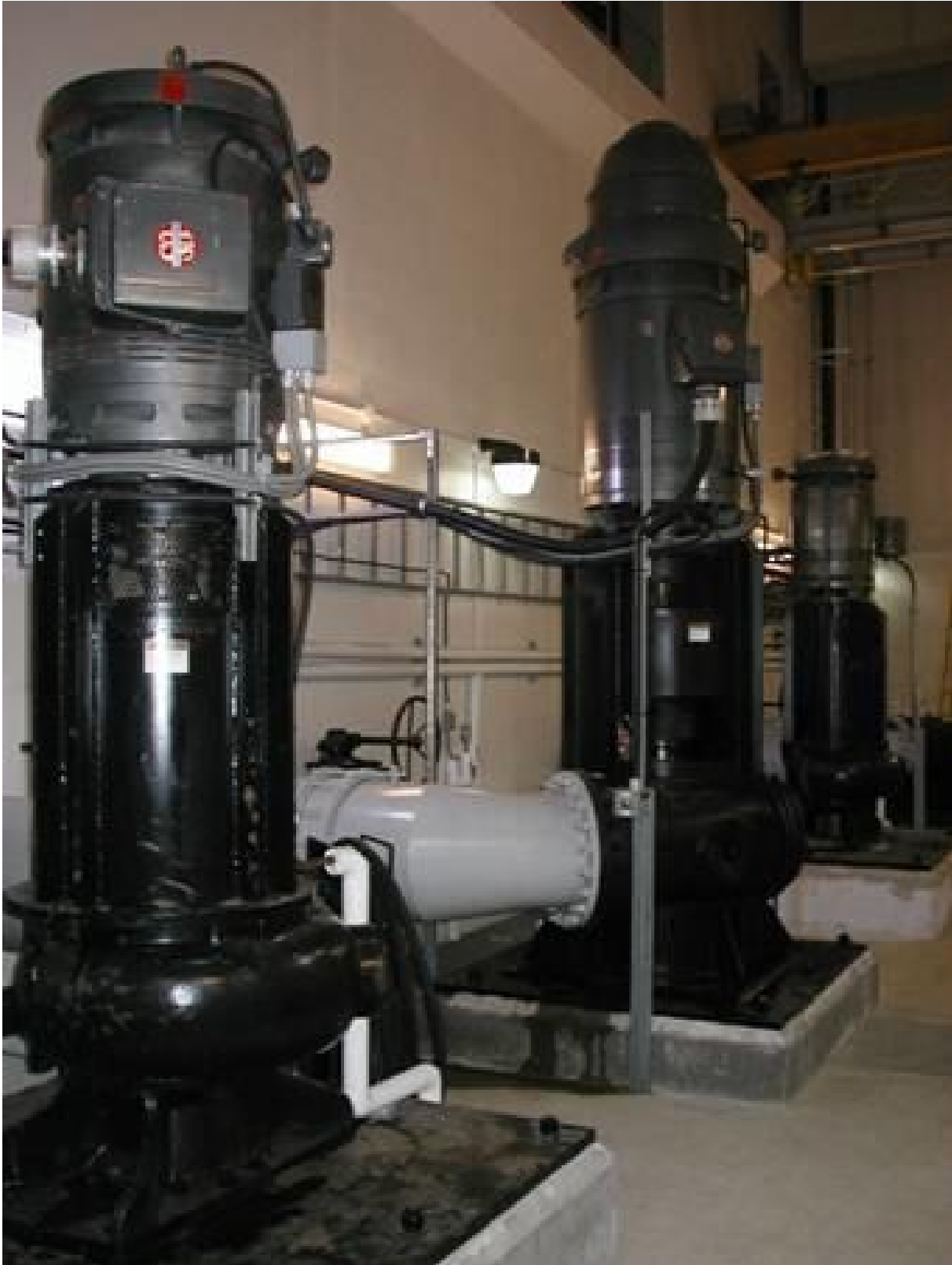
Picture 26 Adelaide Wastewater Treatment Pumps
