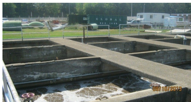
Picture 28 Greenway Section 1 – Crumbling Concrete
