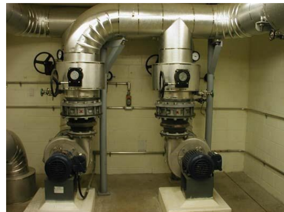
Picture 50 Landfill Exhaust Fans
