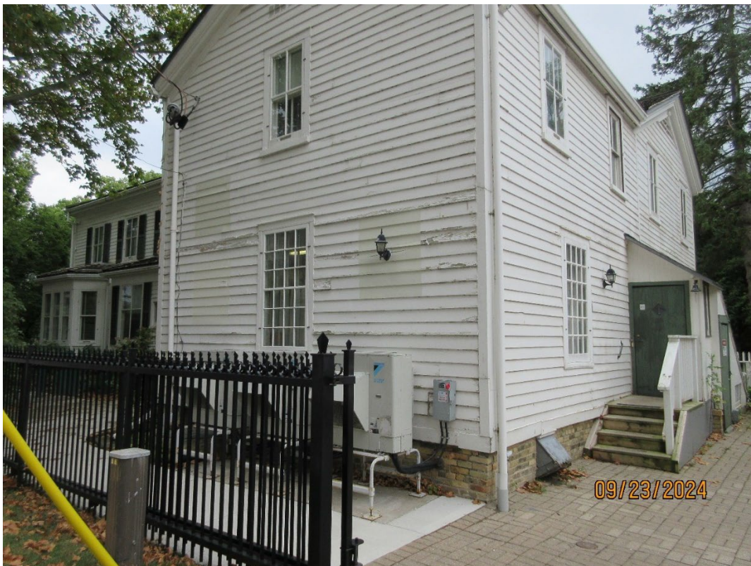
Image 2: Exterior paint test patches on the east exterior wall of the Servants' Quarters at Eldon House.
