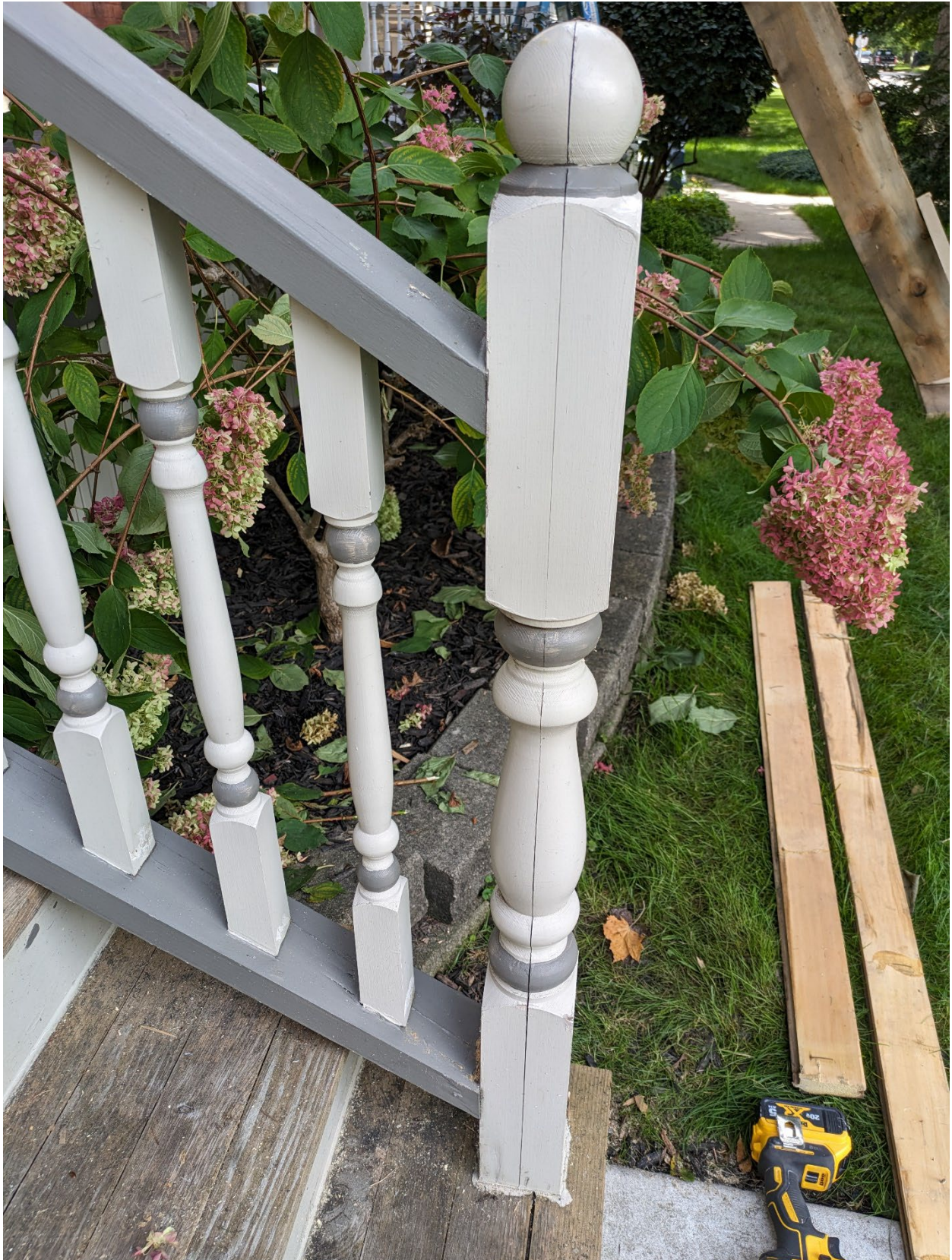
Image 3: Photograph submitted with the Heritage Alteration Permit application demonstrating need for repair or replacement of the post on the front porch steps at 332 St James Street.
