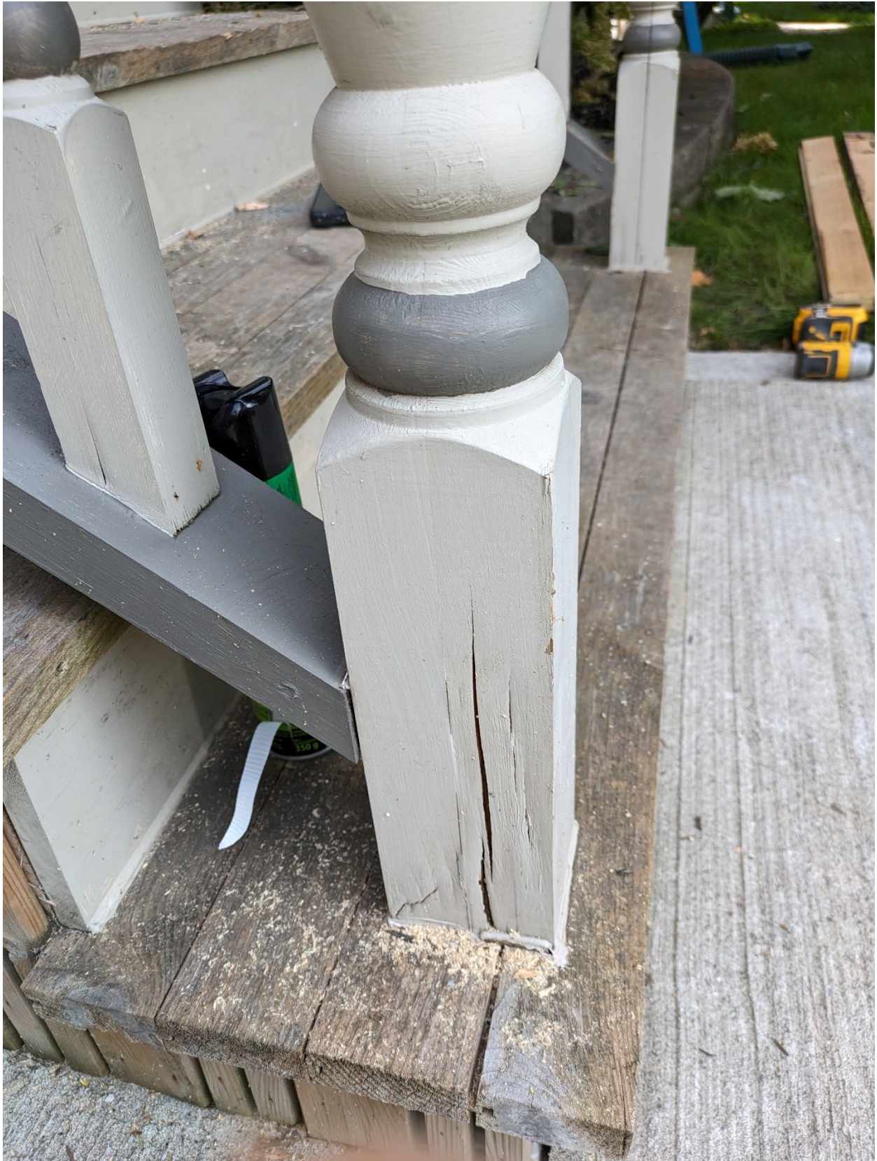
Image 4: Photograph submitted with the Heritage Alteration Permit application demonstrating need for repair or replacement of the post on the front porch steps at 332 St James Street.
