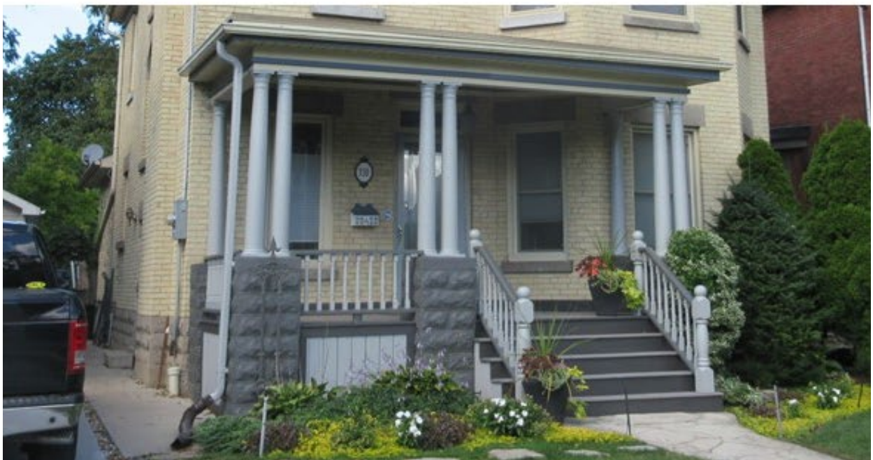
Figure 4: Comparison of porch at 330 St James Street in 2017 prior to replacement without Heritage Alteration Permit approval (top), after replacement in 2020 with vinyl (plastic) materials without Heritage Alteration Permit approval (middle), and after replacement with wood materials in 2021 following Municipal Council's approval of the Heritage Alteration Permit application (bottom).
