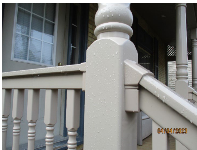
Image 11: Photograph showing detail of the vinyl (plastic) porch materials used for the replacement of the porch at 27 Bruce Street within the Wortley Village-Old South Heritage Conservation District.
