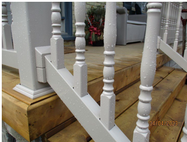
Image 10: Photograph showing detail of the vinyl (plastic) porch materials used for the replacement of the porch at 27 Bruce Street within the Wortley Village-Old South Heritage Conservation District.
