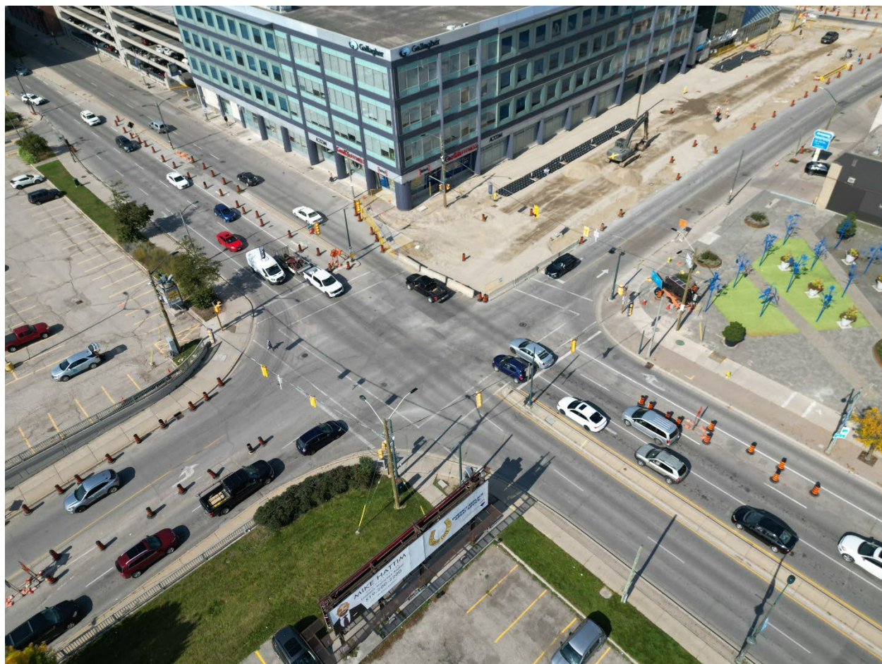
Above: Aerial view of the construction site at Wellington Street and York Street.
