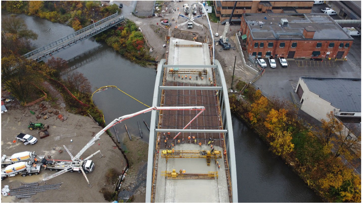
Above: An aerial view of the concrete pouring for the new bridge deck.
