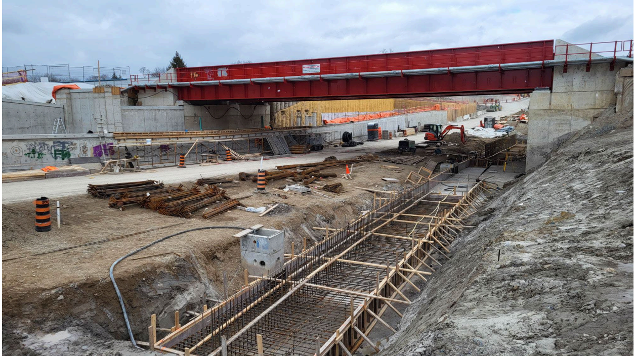
Above: A view of the construction site for the new road under the rail bridge at Adelaide Street North.
