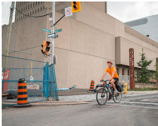
Above: Cyclist crossing the Ridout Street North and Dundas Place intersection adjacent to an active construction zone.
