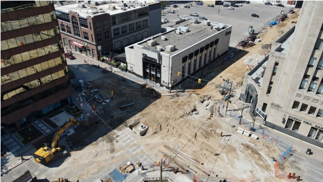
Above: Aerial view of the Downtown Loop Phase 2 construction site at the Queens Avenue and Richmond Street intersection.
