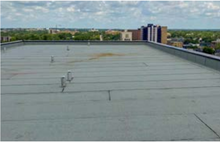
The roof at Kent Street was upgraded to provide enhanced weather resistance and increased energy efficiency, ensuring greater comfort for residents while potentially reducing long-term maintenance costs.
