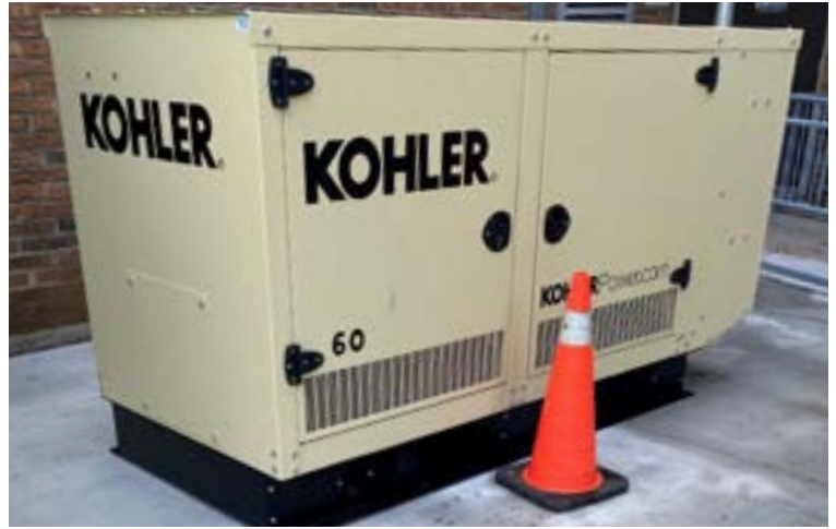
Replacing the generator at Base Line Road will safeguard residents' safety, comfort, and help keep essential services such as emergency lighting and heating running during an outage.
