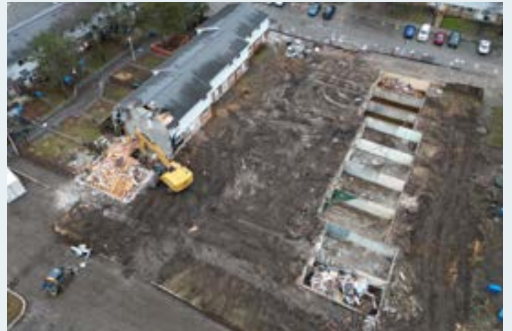
An overhead view at Southdale as 18 units were demolished to make way for the Phase One building, adding 53 purpose-built units to this family site.
