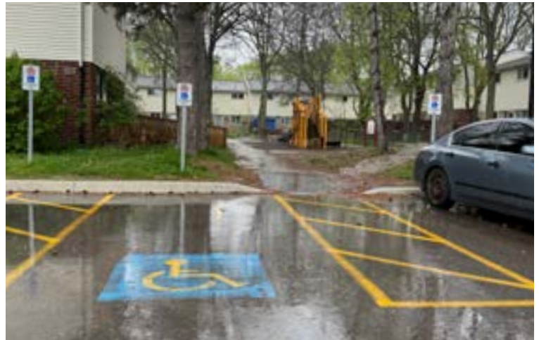
Repaving the roadways and parking lots at Limberlost enhances safety and aesthetics, providing smoother driving surfaces and creating a more welcoming environment.
