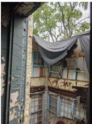
Photo 14: East porch collapse in June 2021
