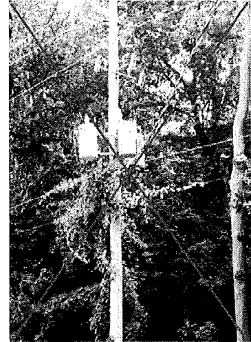
Pole growth contacting electrical equipment & powerlines
