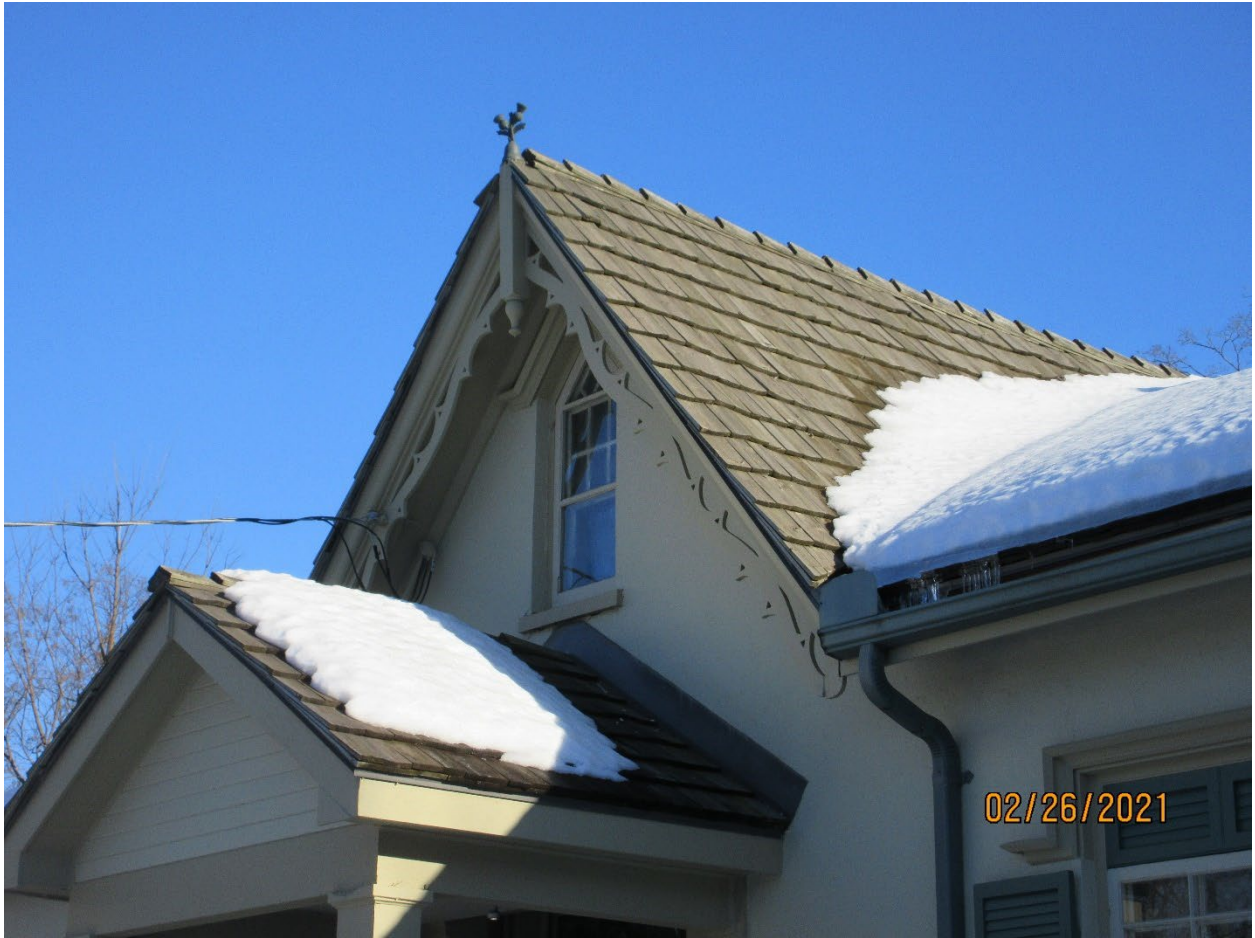
Image 25: View of the central gable dormer on the front (north) facade of Carfrae Cottage with a primitive Gothic pointed wood window. The decorative wood bargeboard of the central gable dormer is also shown, as well as the Scotch thistle (2021).
