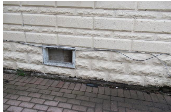
Photo Exhibit No. 11 28 Wellington – exterior façade bricks extend below grade but support the bricks above.
