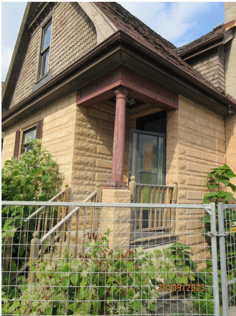
Image 6: Photograph showing part of the building on the subject property at 30 Wellington Road (taken September 20, 2023).
