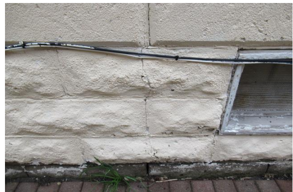
Photo Exhibit No. 6 28 Wellington – cracking through bricks.
