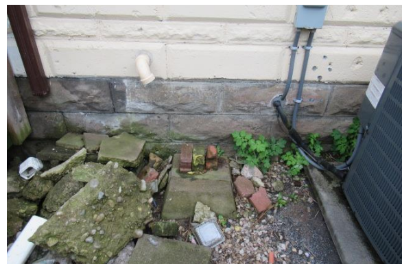
Photo Exhibit No. 12 28 Wellington – exterior façade bricks extend below grade but support the bricks above.
