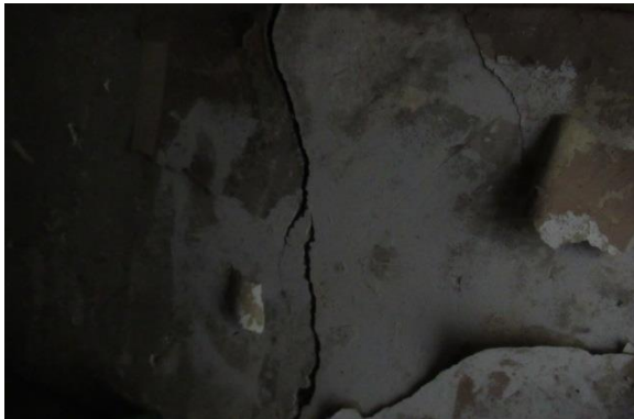
Photo Exhibit No. 20 30 Wellington – large cracks in the stairwell concrete wall.
