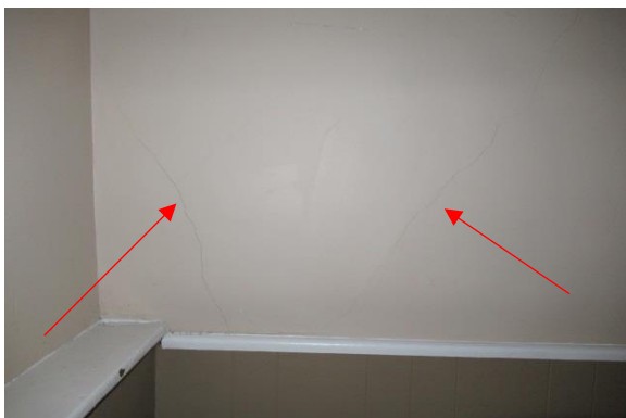
Photo Exhibit No. 9 28 Wellington – large cracks extending full wall height in stairwell walls.
