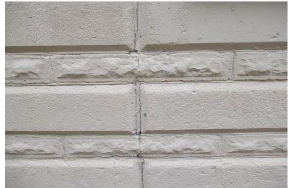
Photo Exhibit No. 5 28 Wellington – cracking through bricks.
