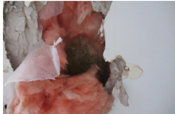
Photo Exhibit No. 17 30 Wellington – substantial amount of moisture in exterior walls.
