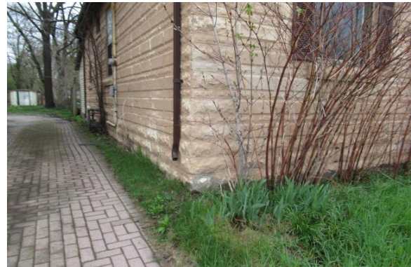
Photo Exhibit No. 23 30 Wellington – exterior façade bricks extend below grade but support the bricks above.
