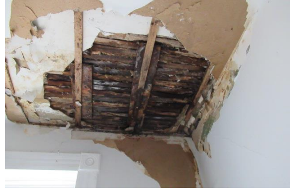
Photo Exhibit No. 16 30 Wellington – substantial water damage on the interior.
