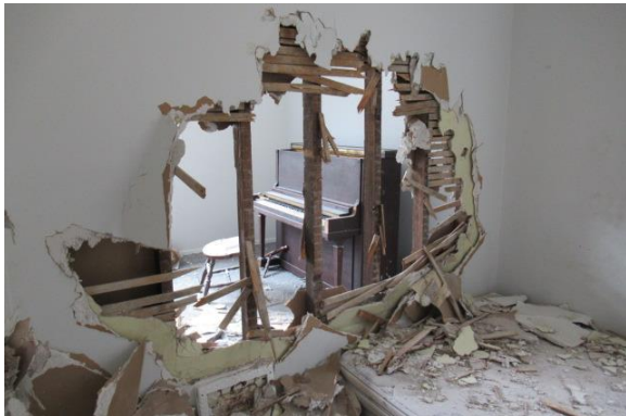
Photo Exhibit No. 14 30 Wellington – substantial interior damage.
