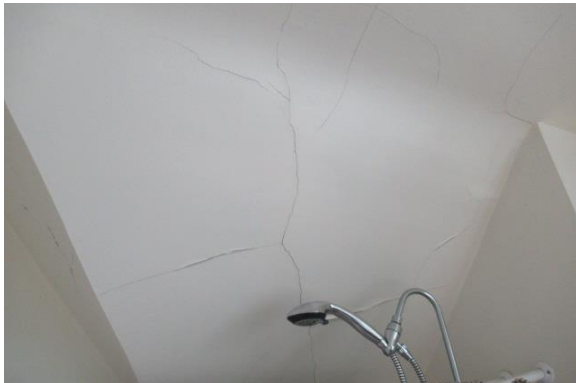
Photo Exhibit No. 8 28 Wellington – large cracks extending full ceiling length in upper-level ceiling.
