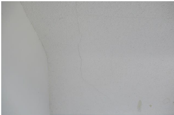
Photo Exhibit No. 21 30 Wellington – large cracks in the ceiling, extending full ceiling length.
