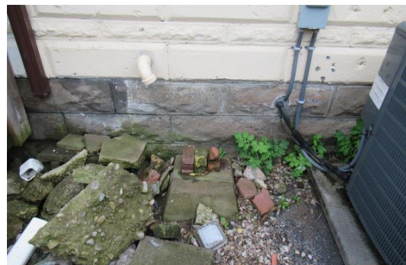
Photo Exhibit No. 12 28 Wellington – exterior façade bricks extend below grade but support the bricks above.
