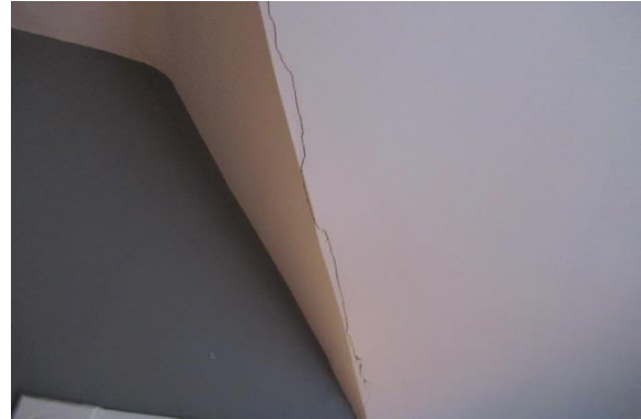
Photo Exhibit No. 10 28 Wellington – large cracks extending full ceiling length in upper-level ceiling.
