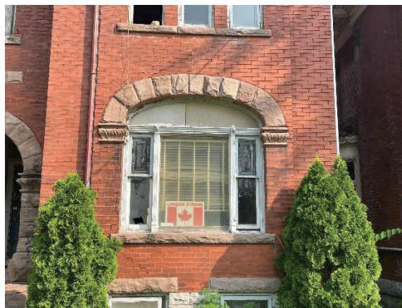
Photo 19: First storey of the eastern bay of the front façade, looking north
