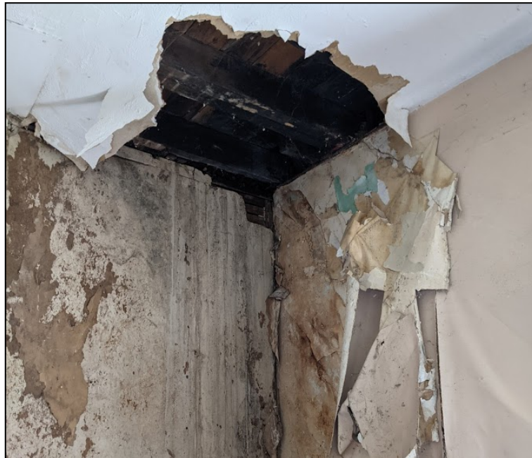
Photograph 1 - Interior finish damage
