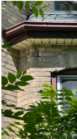
84. 7056 Pack Rd Brick Damage.HEIC
