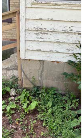
85. 7056 Pack Rd Cracked Cinder Block Mudroom Foundation.HEIC
