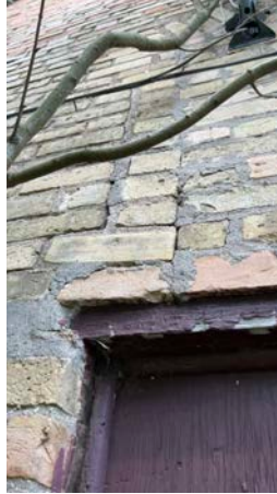
95. 7056 Pack Rd Mortar Damage 1.HEIC
