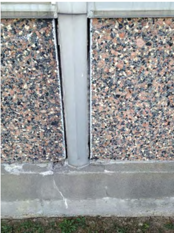
Caulking missing at precast panels - East Elevation
