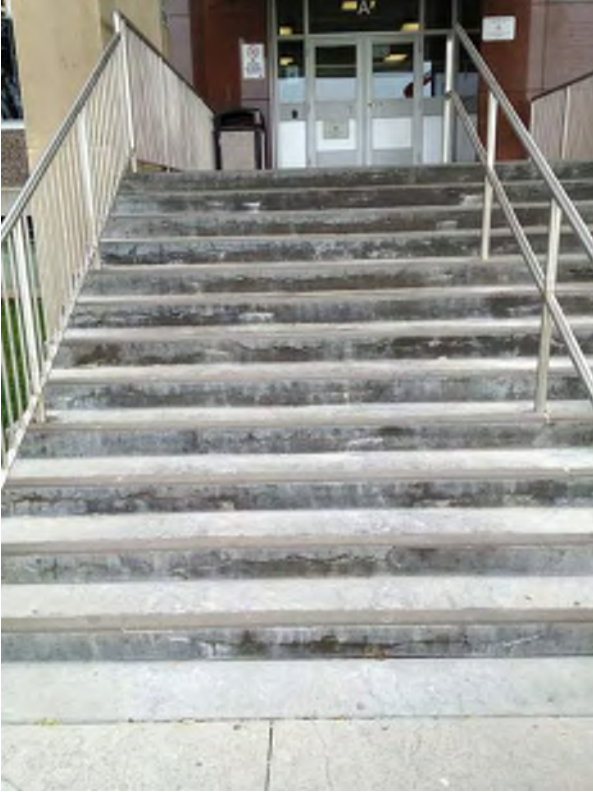
Existing front entry stairs and sidewalks have been replaced in the last decade, yet show signs of damage and wear. Intermediate handrail spacing does not comply with current building code
