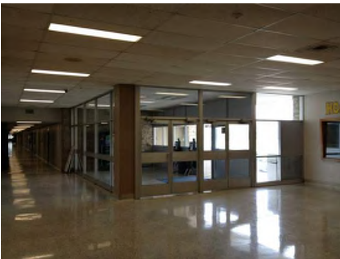
Fire exit sign missing from rear exit
