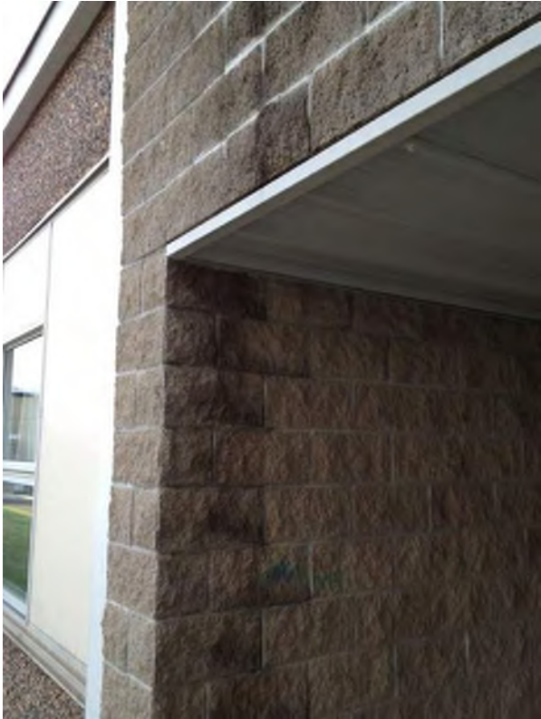
Water damage at soffit - East Elevation 1988 addition
