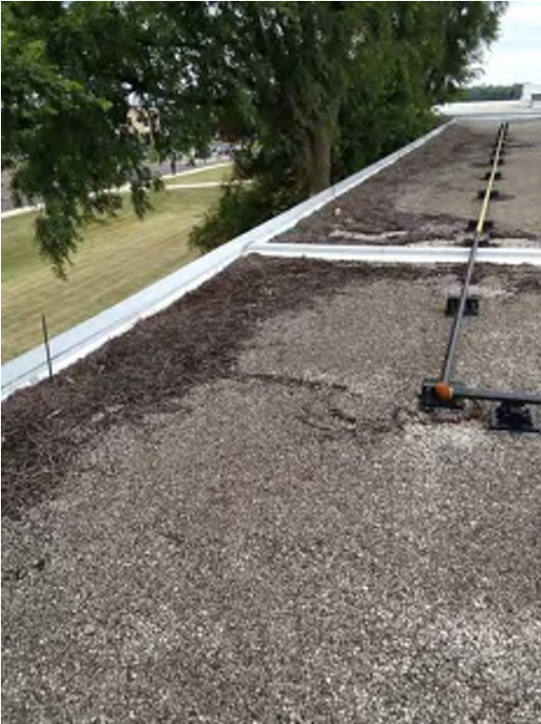
Debris at overhanging trees on Roof H
