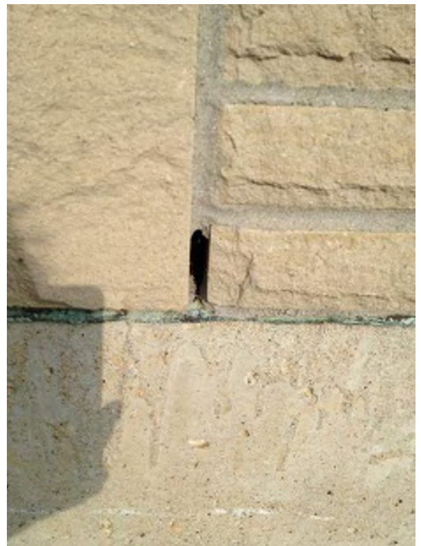
Missing brick vents - 1988 addition
