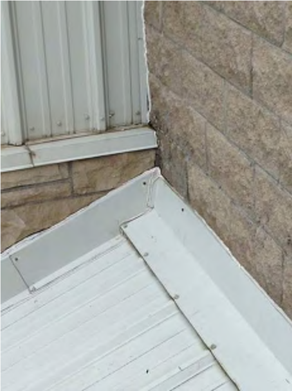
Water damage at concrete block causing deterioration of mortar joints - North Gymnasium Elevation
