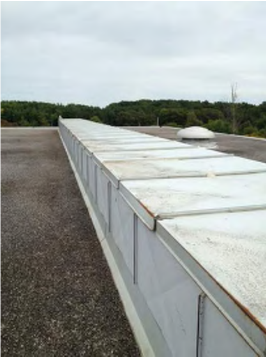
Metal flashing over ductwork above gymnasium beginning to rust - finish has deteriorated
