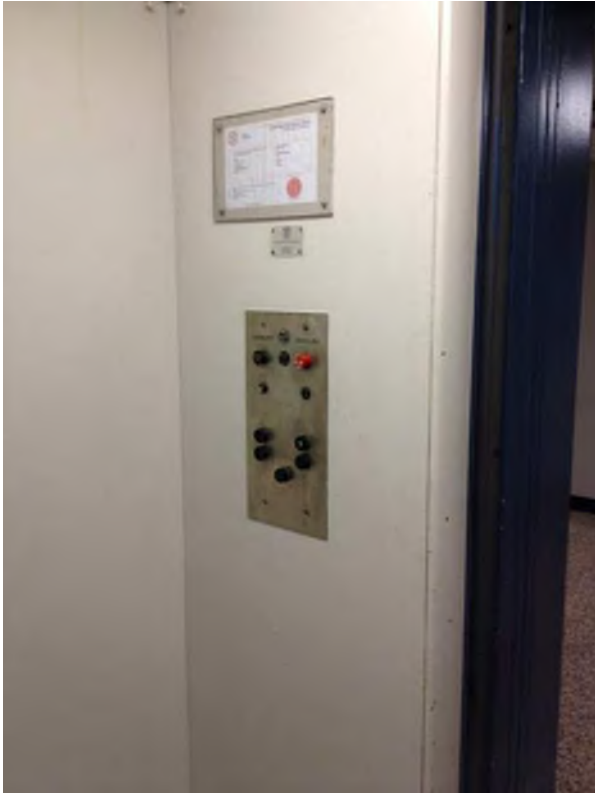
Elevator interior cab panel
