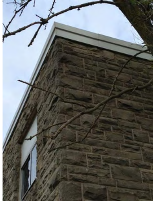
Deteriorated mortar joints at upper stone - Tech Wing
