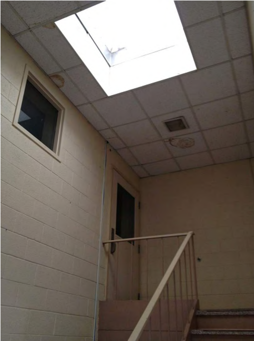
Acrylic Dome Skylight Interior
