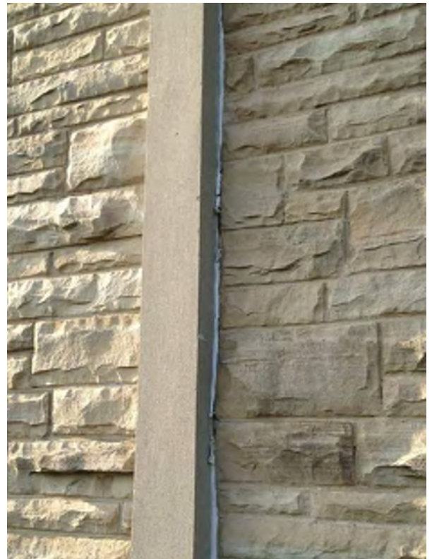
Caulking joint at Gymnasium Wall - South Elevation
