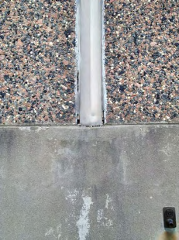
Caulked joint failure on East Elevation.
