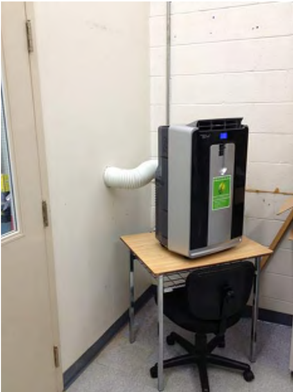
Portable air conditioner
