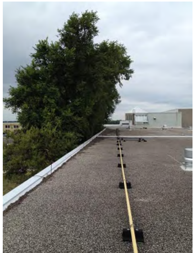
Overhanging trees at Roof H
