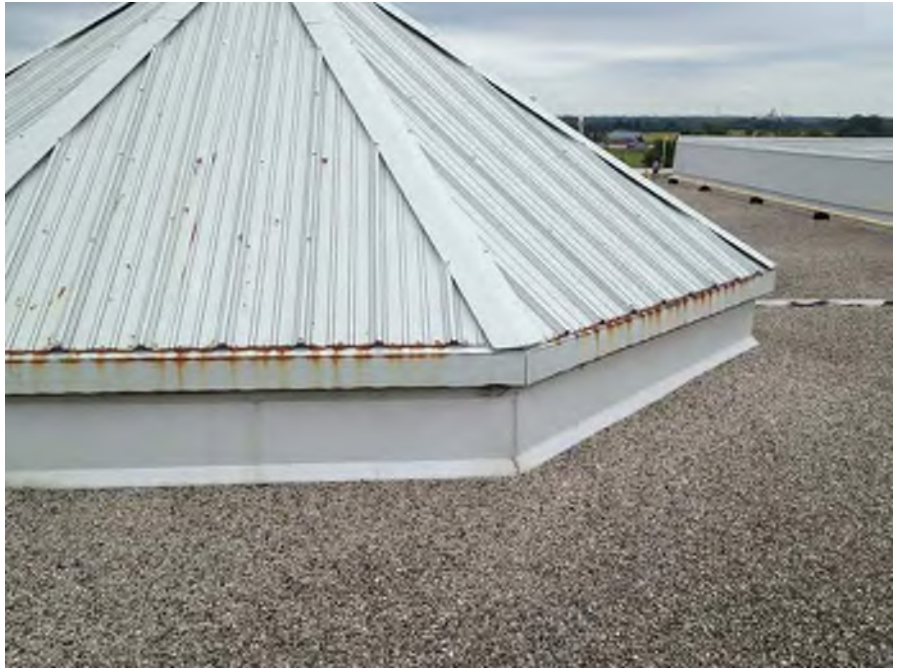
Metal roof over north gymnasium showing rusting
