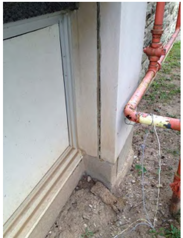
Caulking deteriorated at smooth stone panel - investigation required to view condition of anchors.
