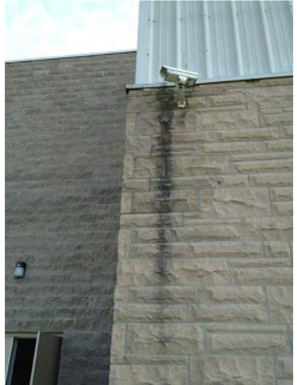
Water Stain from flashing - North Elevation 1988 addition
