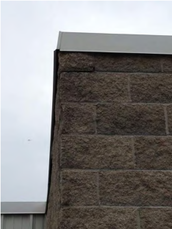
Deteriorated mortar joints at upper corner of 1988 Gymnasium addition.
