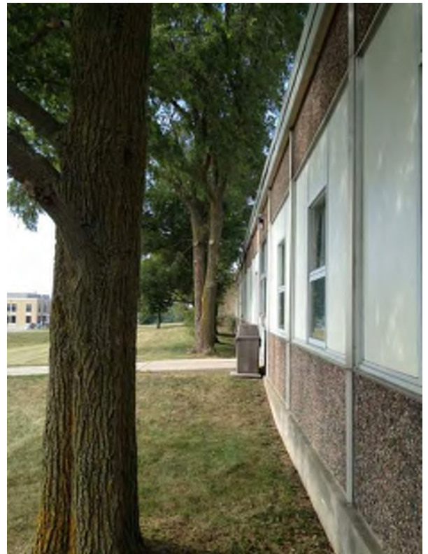
Trees at West Elevation too close to building.
