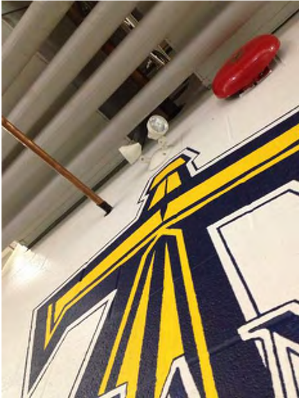
Firestopping missing at pipe penetration.
