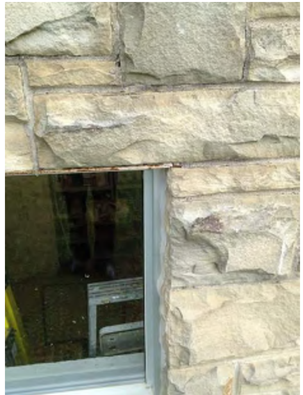
Deteriorated mortar joints and rusting steel lintel at window head.
