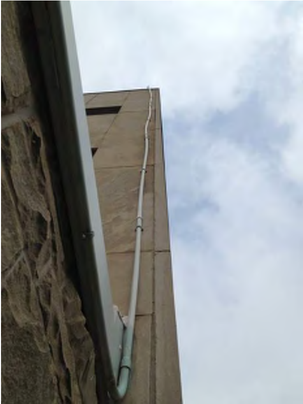
Deteriorated mortar joints at South Elevation
