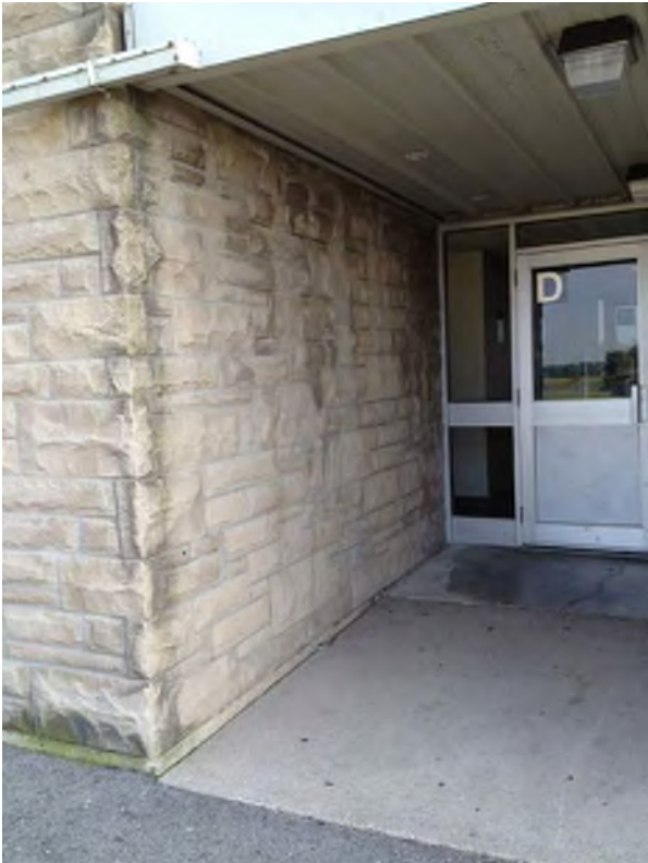
Water damage below soffit - North Elevation 1988 addition
