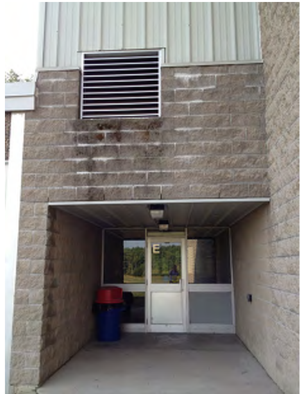
Damage to concrete block masonry from missing metal flashing and sill.
