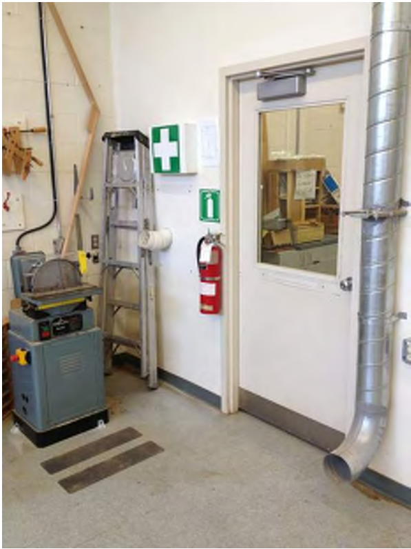
Fabrication Room showing portable air conditioner exhausting into room.
