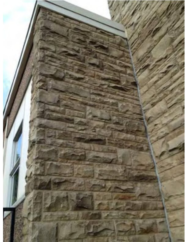
Deteriorated mortar joints on West Elevation.
