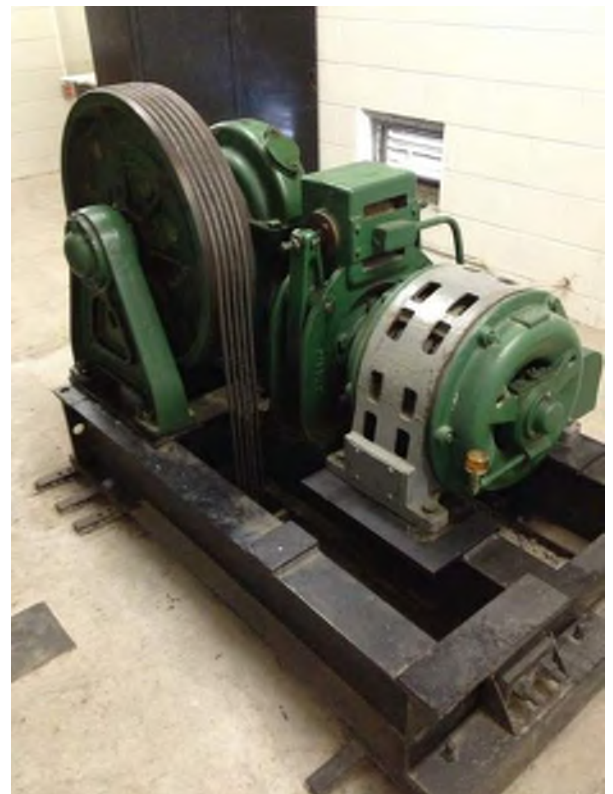
Elevator Machine Room Equipment
