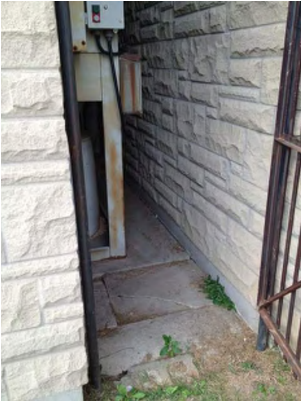
Dust collector enclosure access.
