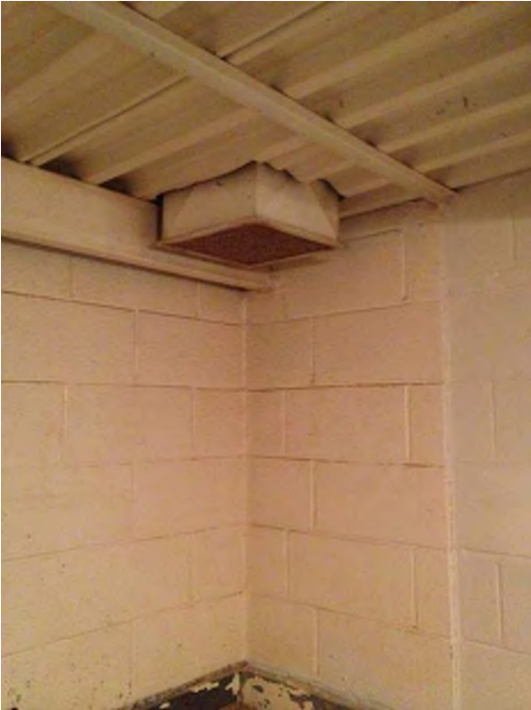
Construction Technology Classroom Finishing Room exhaust vent.
