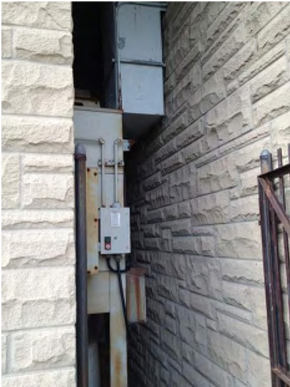
Dust collector enclosure
