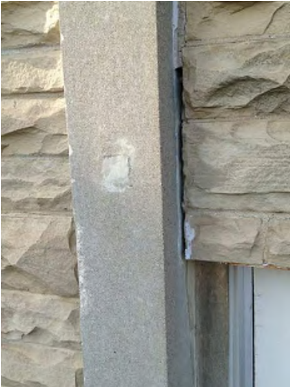
Caulked joint at Gymnasium wall window head - South Elevation. Note deterioration of mortar joints
