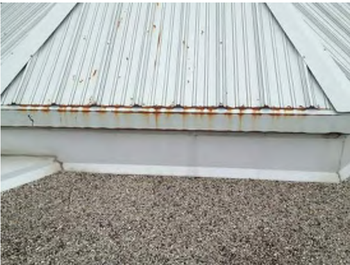
Metal roof over north gymnasium showing rusting
