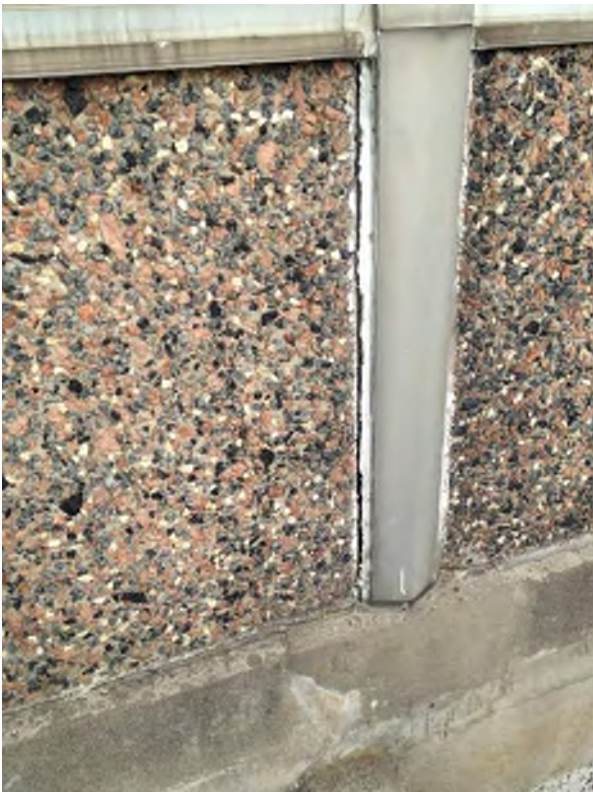
Caulked joint failure on West Elevation.
