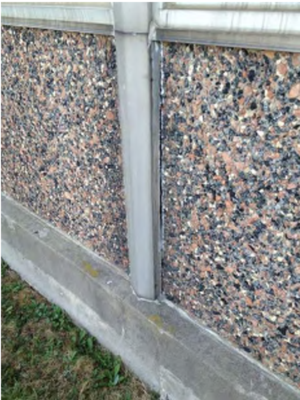
Caulked joint failure on East Elevation
