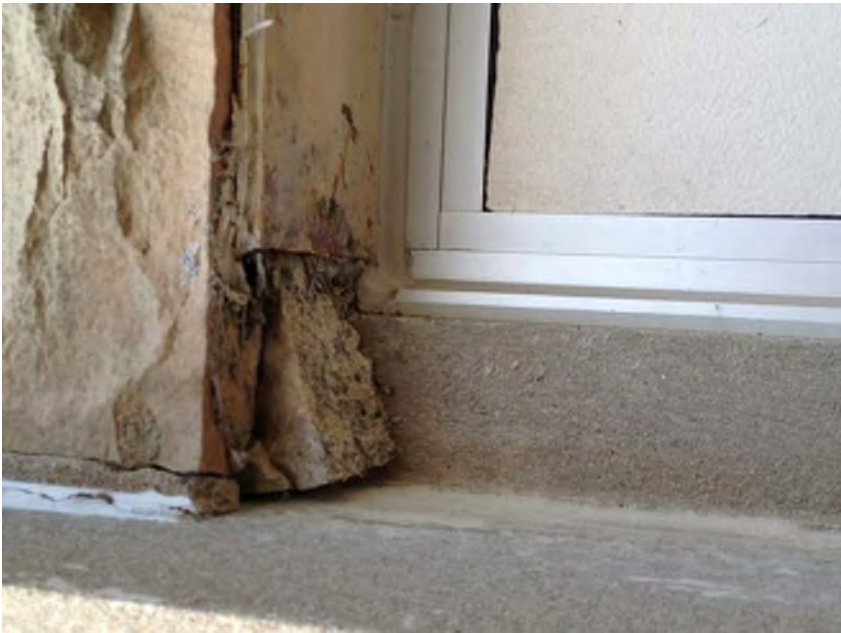
Damage to stone of South Elevation of Gymnasium from moisture at penetration.
