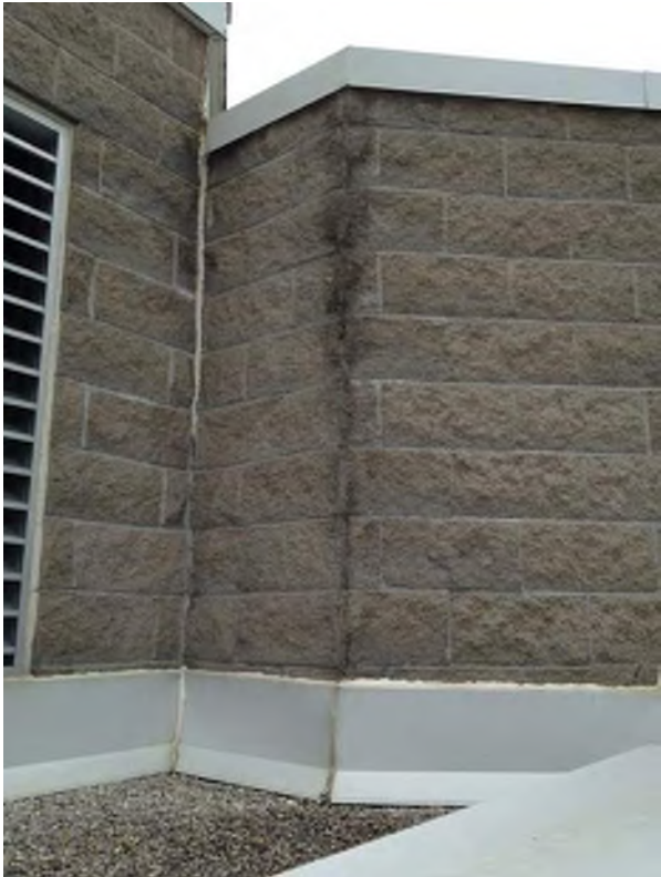
Water damage at concrete block - Upper North Gymnasium Elevation
