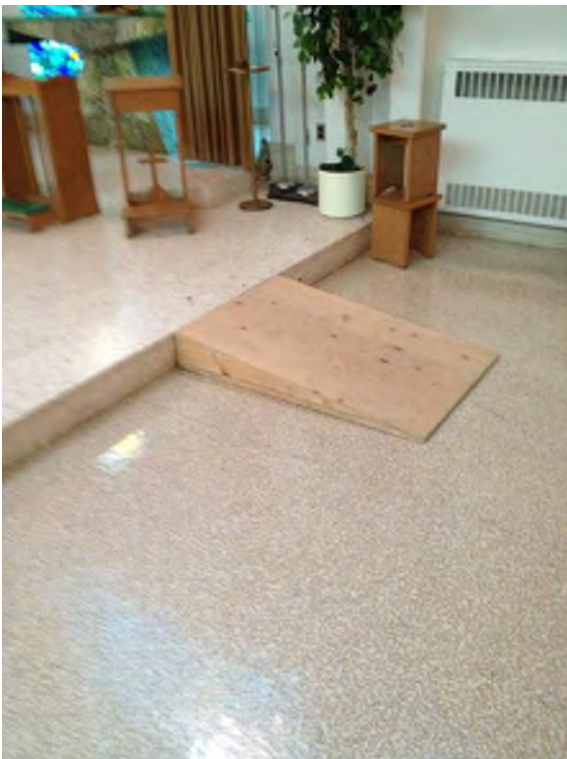
Construction and Installation of wood frames in chapel providing access to sanctuary do not meet current building code requirements for accessibility
