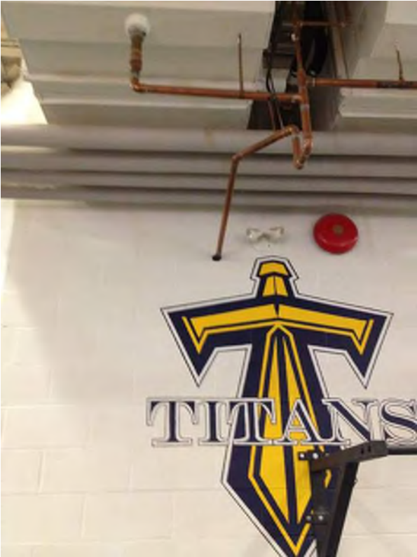
Firestopping missing at pipe penetration.
