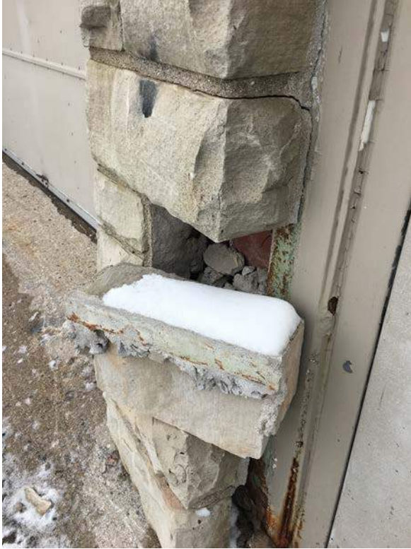
Dislodged stone on pier, at east elevation of Technology Wing (ERA, 2018).
