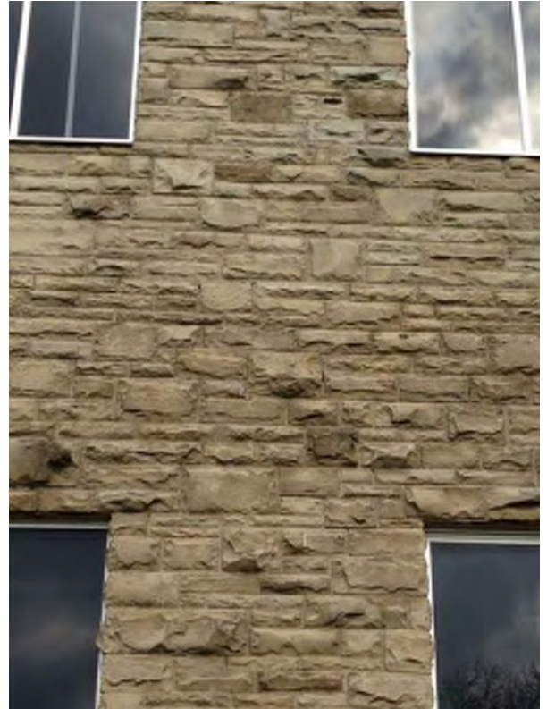
Deteriorated mortar joints below window sill on West Elevation.
