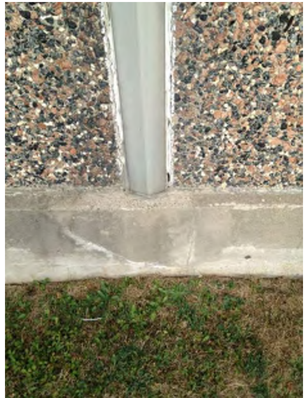
Caulked joint failure on West Elevation.
