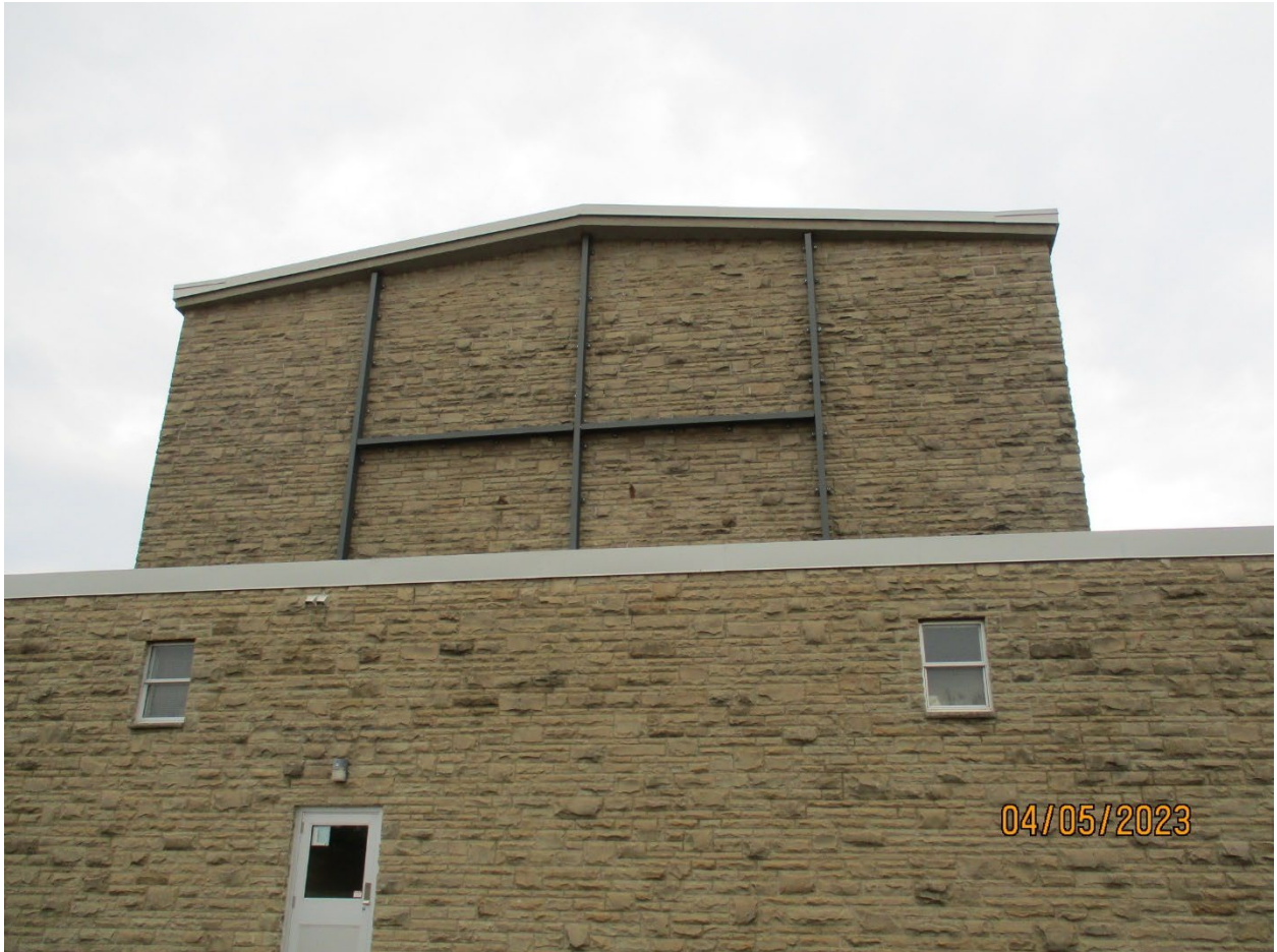
Image 5: Photograph showing stone exterior on the rear of the chapel at Regina Mundi Catholic College.
