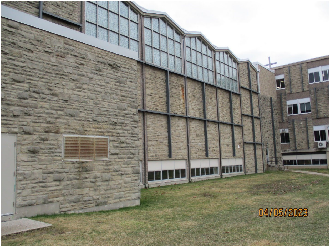
Image 6: Photograph showing stone exterior on the rear of the chapel at Regina Mundi Catholic College. Note the steel bracing observed on the exterior of the school is an interim protection measure.
