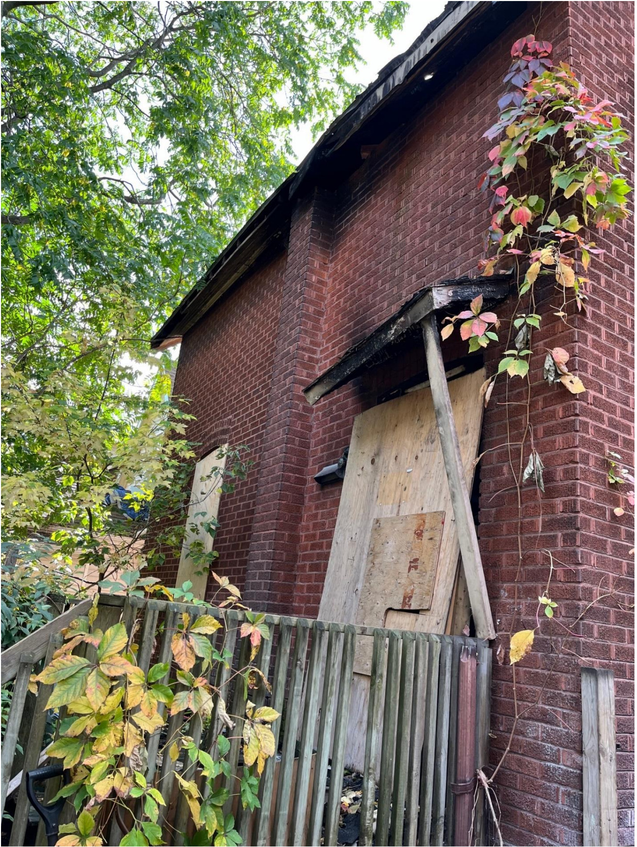
712 Adelaide St N – Rear Exterior w. Fire Damage
