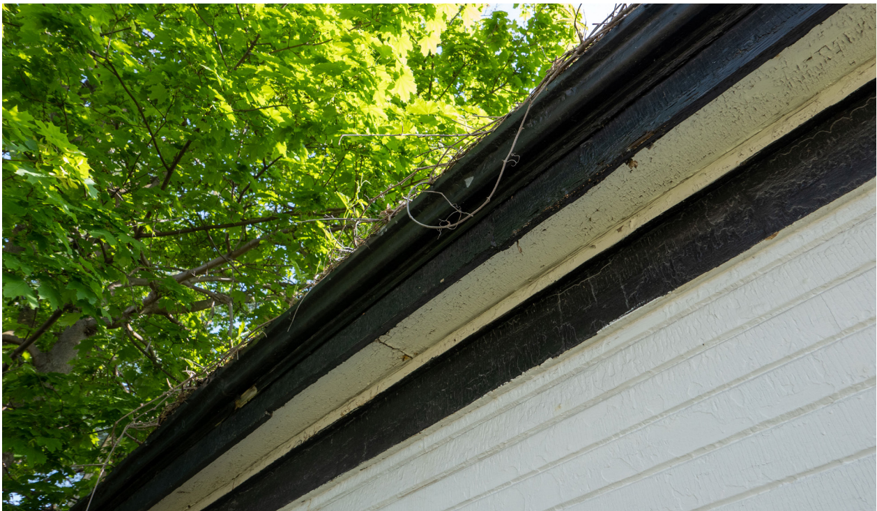
Figure 16: Detail of white soffit and black fascia boards as seen on the west elevation (CBCollective, 2023).
