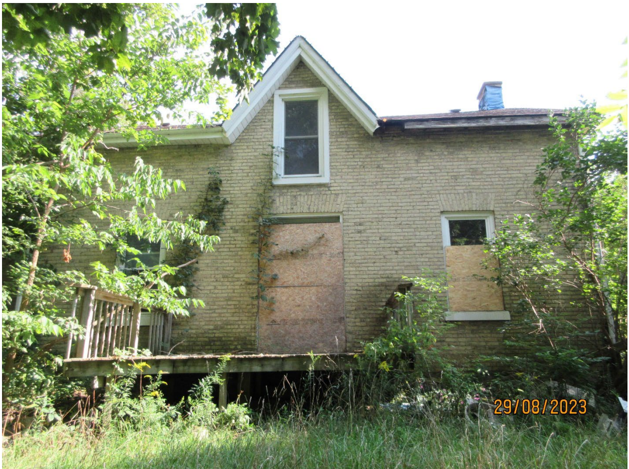
Image 7: Photograph showing north elevation of farmhouse noting flat arch brick lintels located above the window and door opening as well as vinyl window in gable (L.Dent, August 29, 2023).
