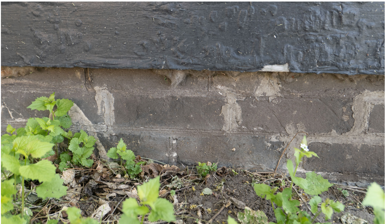
Figure 14: Detail of brickwork on the west foundation, showing re-pointed joints alongside historic pointing with bead tool profile (CBCollective, 2023).
