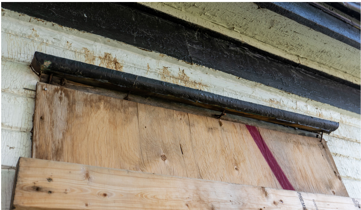
Figure 20: Remnant wooden cornice above the window opening on the west elevation (CBCollective, 2023).
