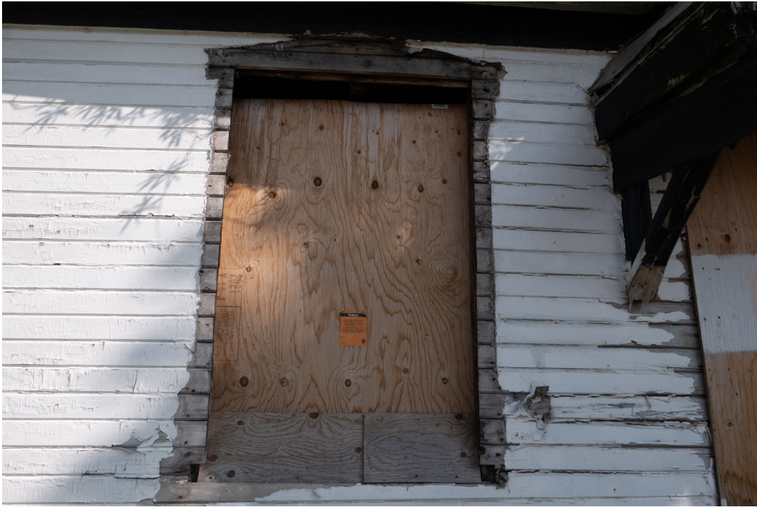
Figure 19: View of the west window opening on the south elevation showing removed window and the former profile of the wood surrounds (CBCollective, 2023).
