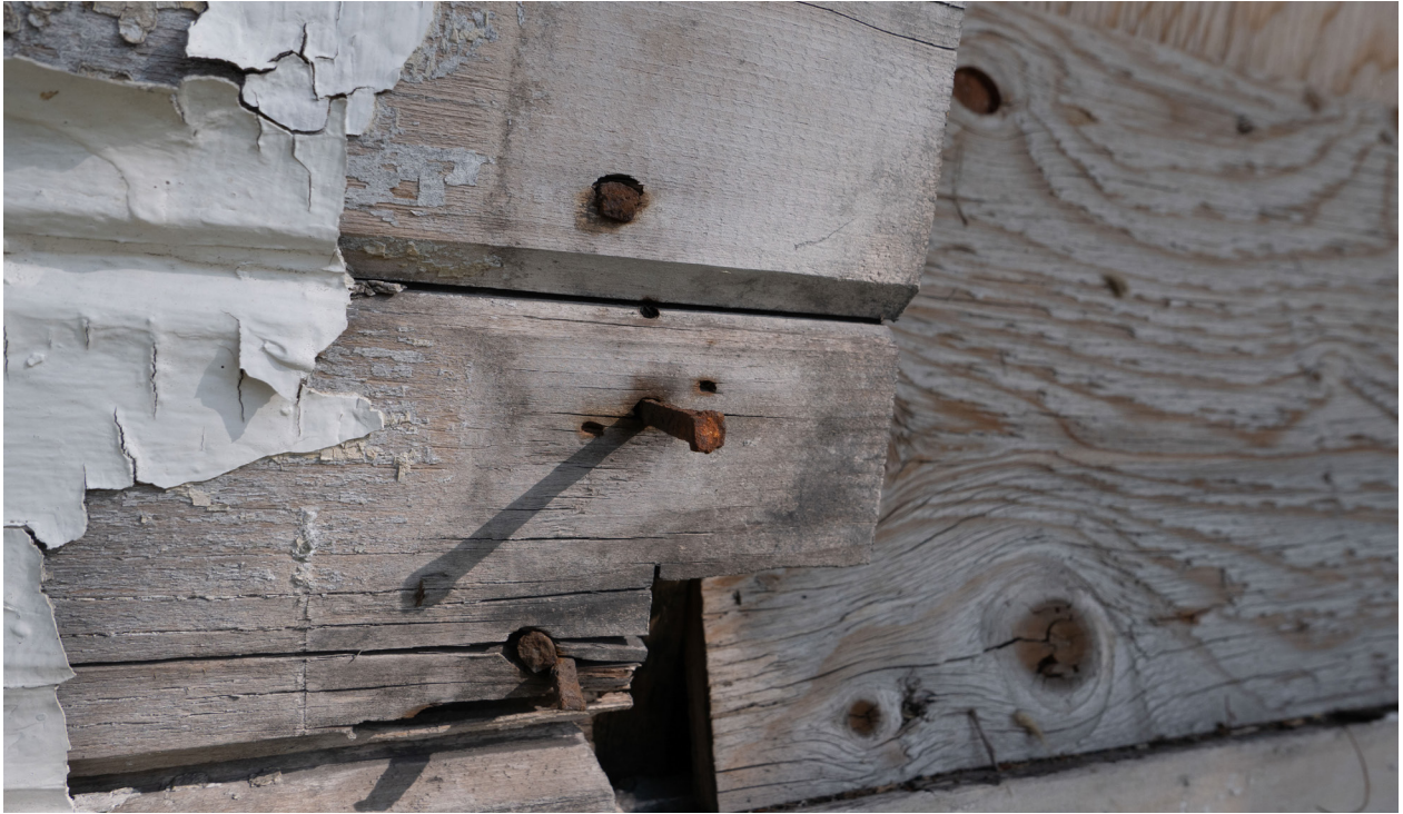
Figure 21: Exposed window openings reveal the use of machine-made nails (CBCollective, 2023).
