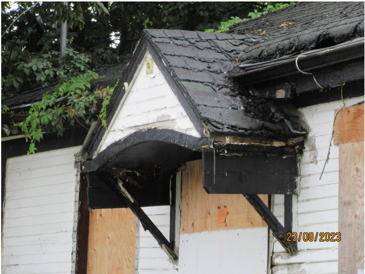
Image 6: Awning on the south elevation of the building on the subject property at 176 Piccadilly Street, August 23, 2023.
