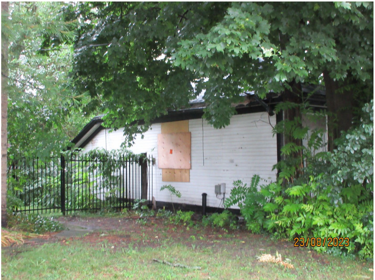
Image 4: North elevation of the building on the subject property at 176 Piccadilly Street, May 2, 2022.
