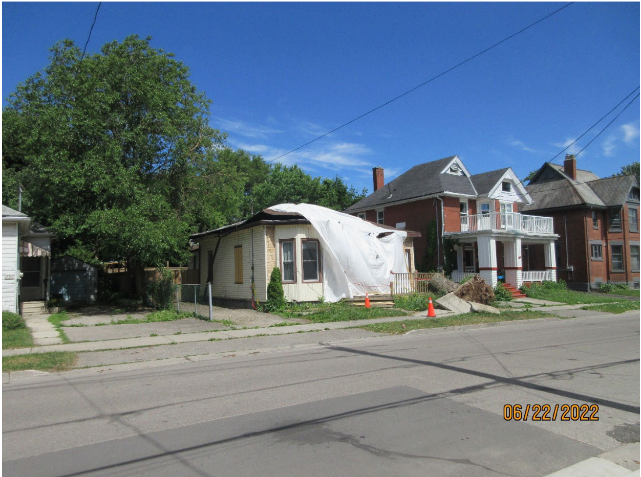
Image 1: Photograph of the former house previously located on the subject property at 520 Ontario Street following extensive tree damage, June 22, 2022.
