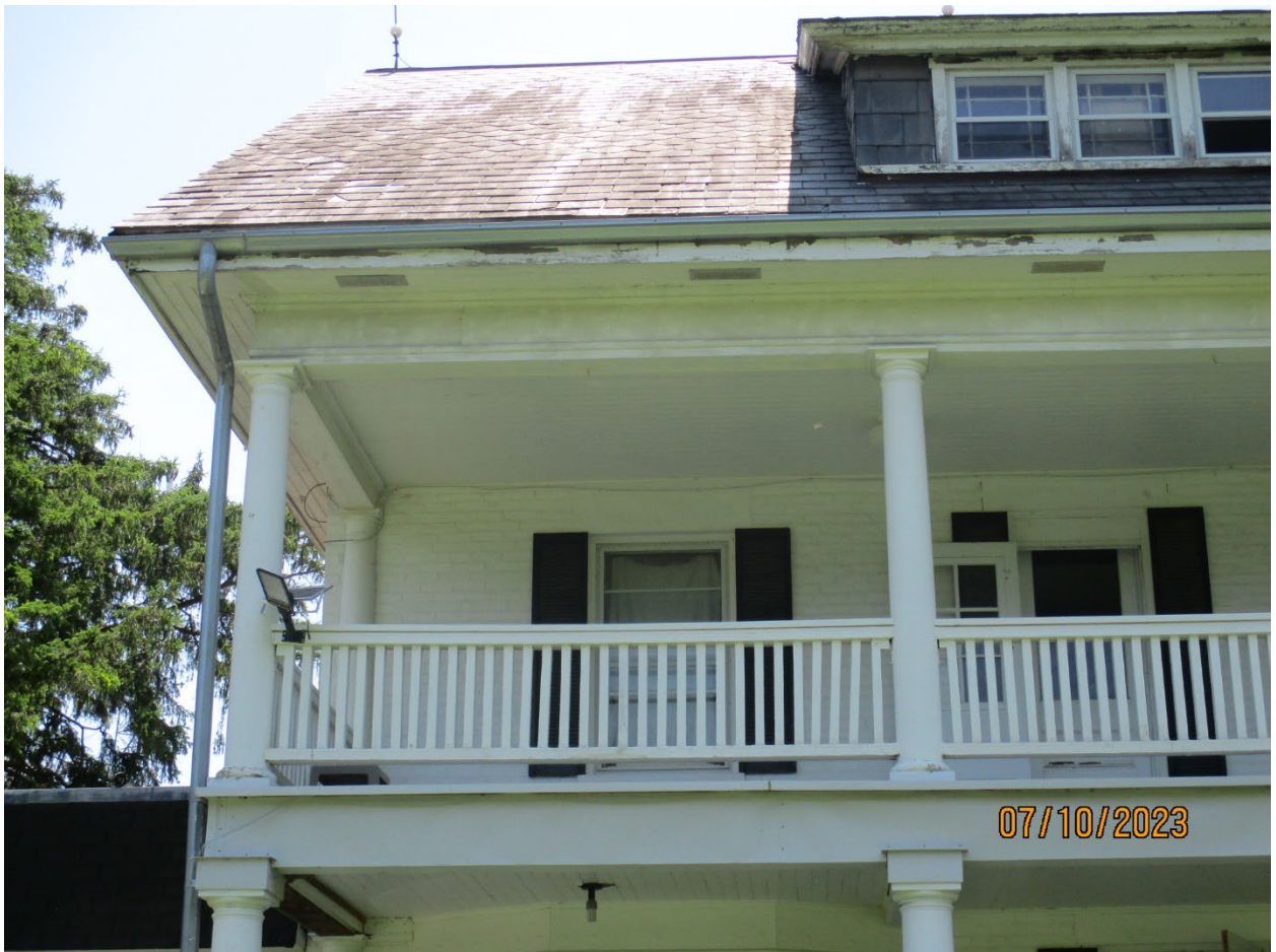
Image 4: Photograph showing the slate roof, shed roof dormer, frieze, and second storey porch details.
