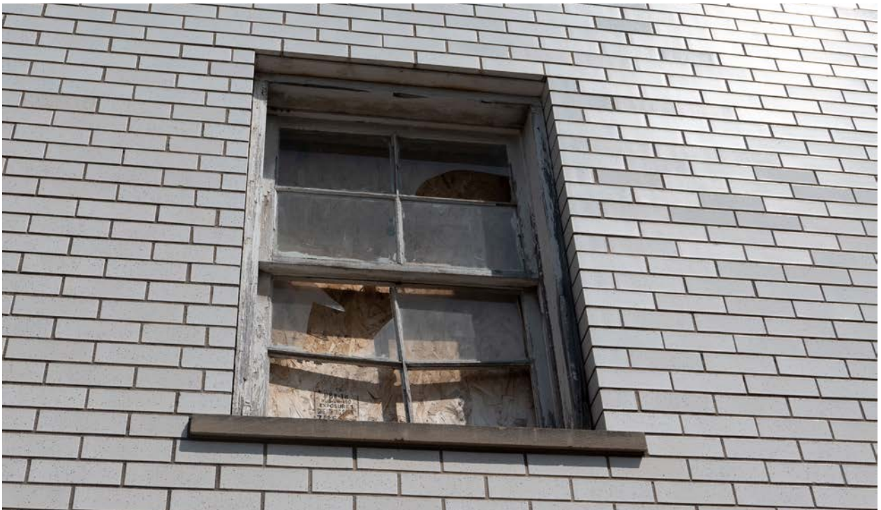
Figure 8: Remnant four-over-four wooden sash window on the south elevation, in poor condition (CBCollective 2023).
