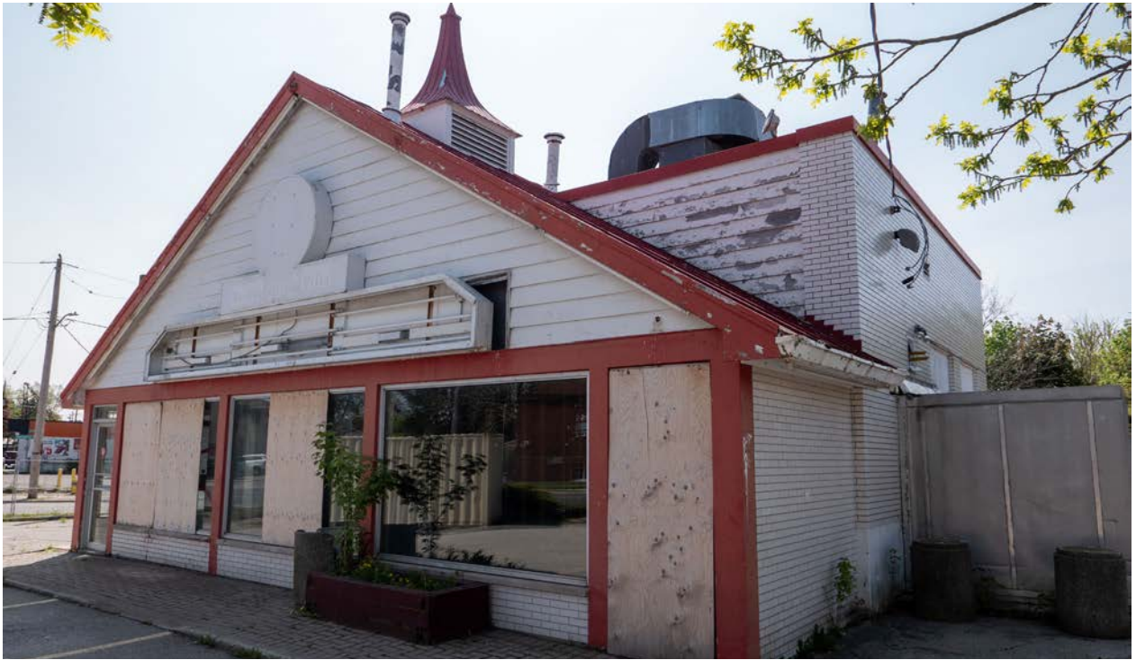
Figure 7: Southwest view of the building's north elevation, including the gabled addition, and siding applied to the original mass (CBCollective 2023).
