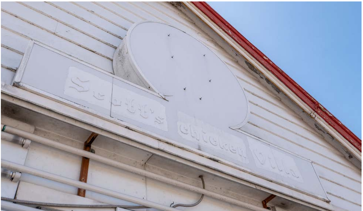
Figure 12: Two remnant signs on the front of the building, including ghosted text when the location was branded a Scott's chicken Villa (CBCollective 2023).
