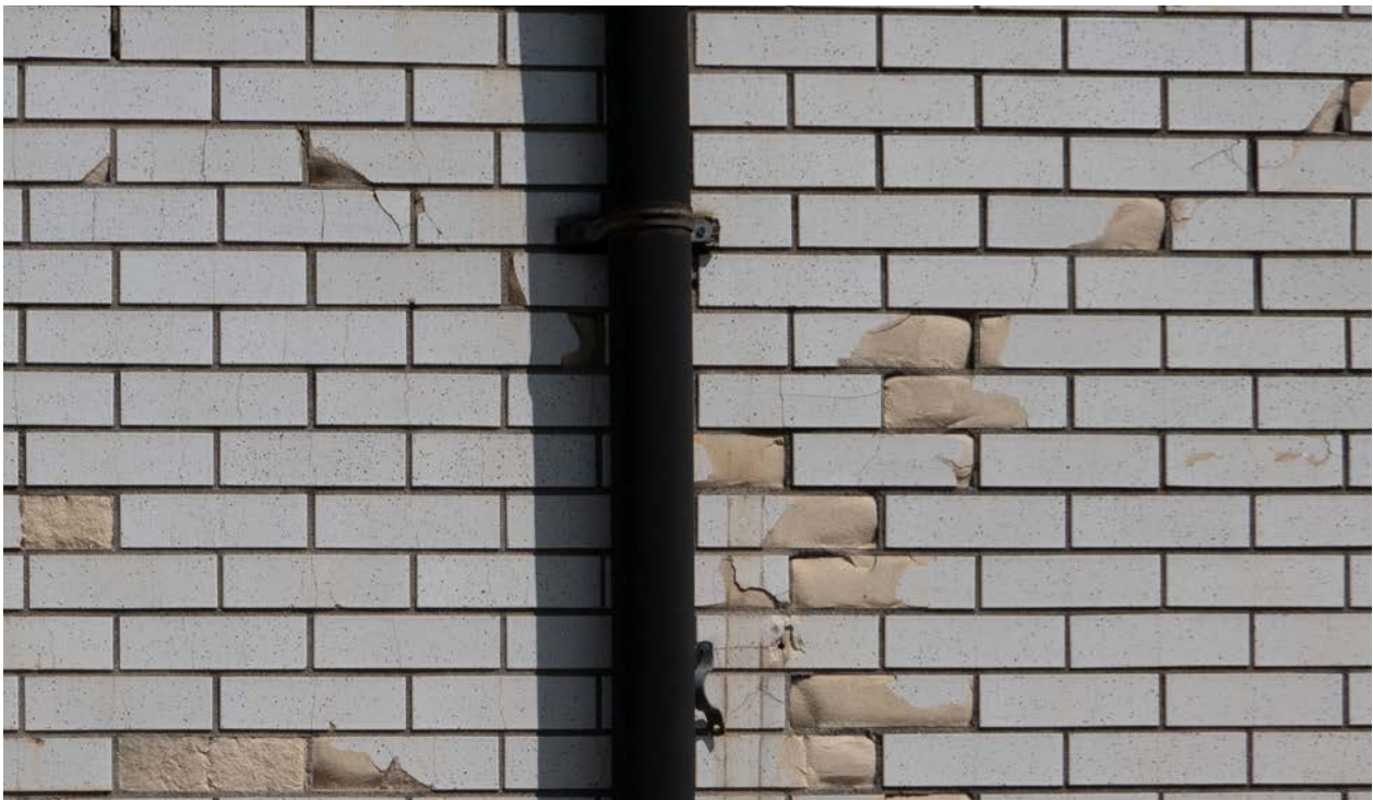
Figure 10: Detail of speckled white enamel brick on the south elevation, with damage revealing buff material beneath (CBCollective 2023).
