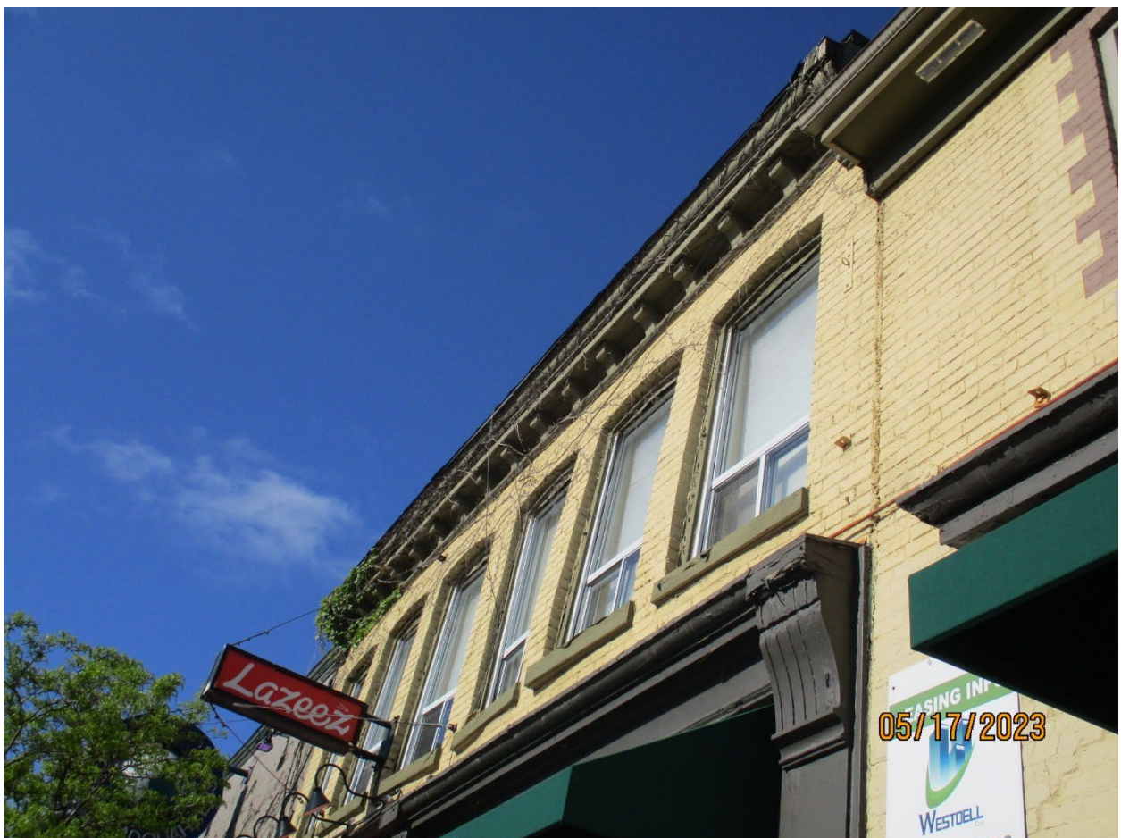
Image 2: Photograph showing second storey windows on the upper facade of the building at 599 Richmond Street.
