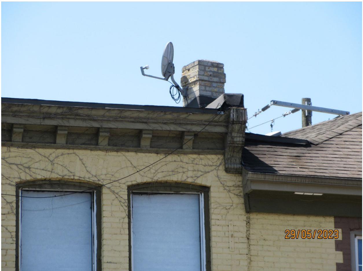
Image 4: Photograph showing roofline, cornice, corbel, and bracket details on the building at 599 Richmond Street.
