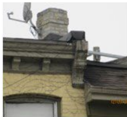
5. Cornice details including a) large corbels on each end of the cornice, and b) smaller band of corbels spanning the entirety of the east cornice.
