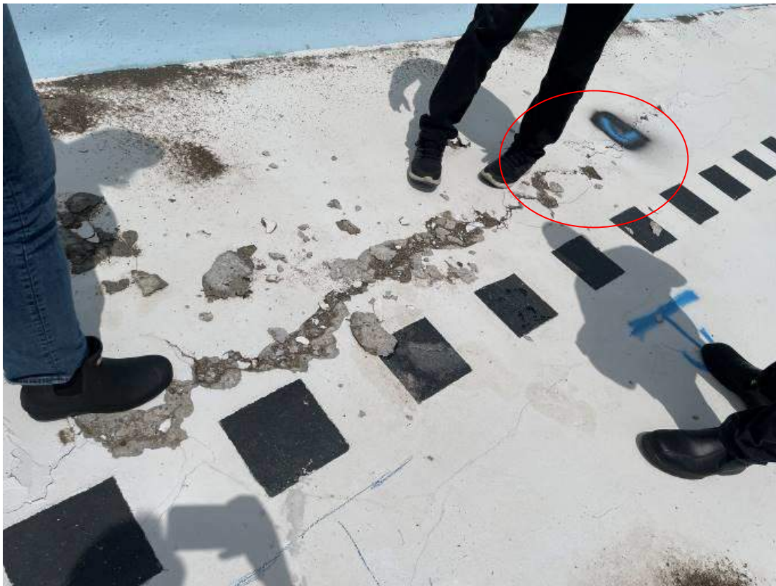
Figure 2a – Significant fracture in lane 1 at break point to deep area (June 2022)
