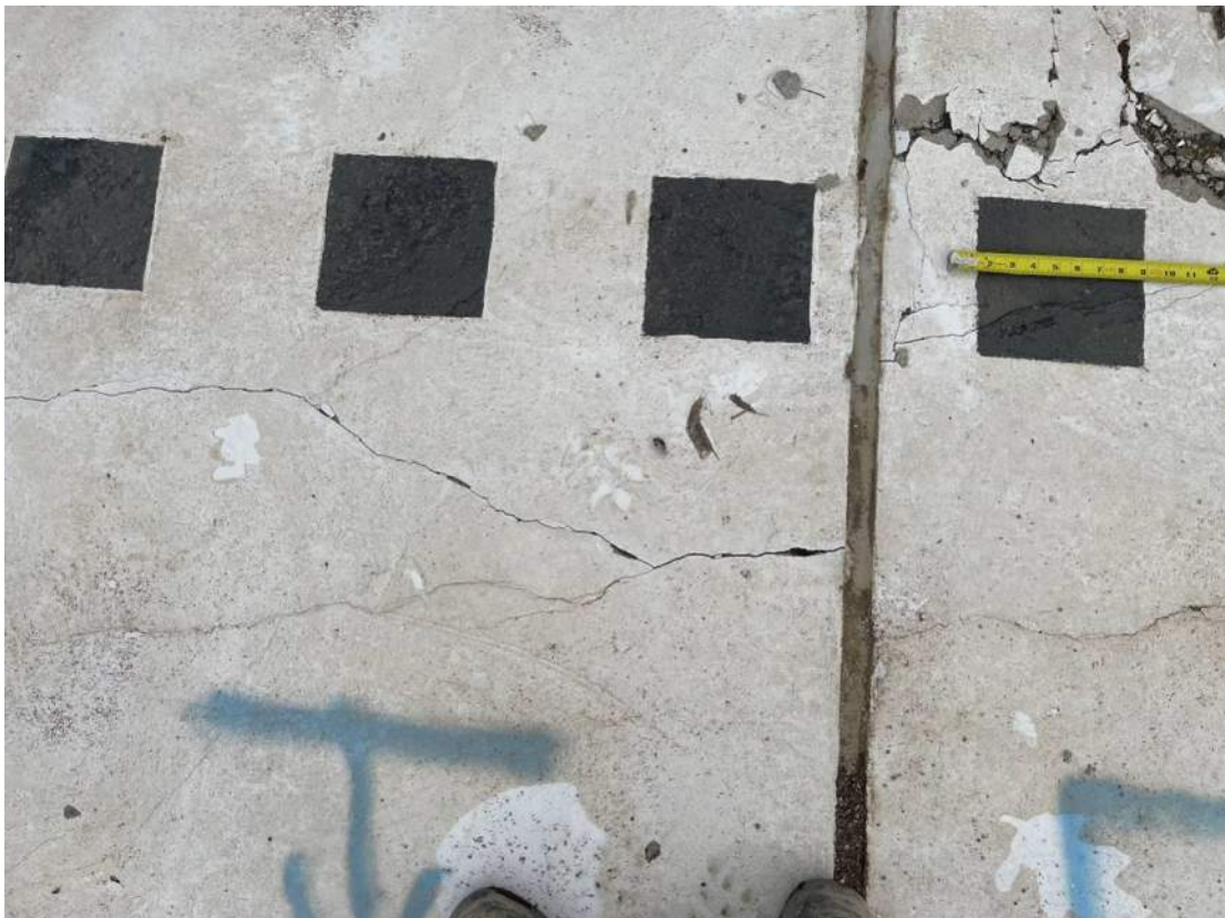
Figure 4b – Fracture in lane 1 at break point to deep area (April 2023)
