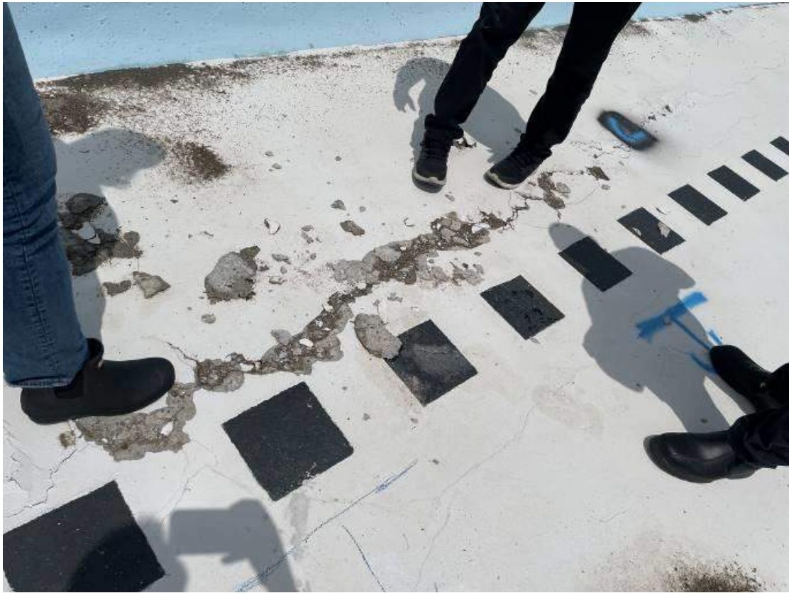
Figure 2 – Significant fracture in lane 1 at break point to deep area
