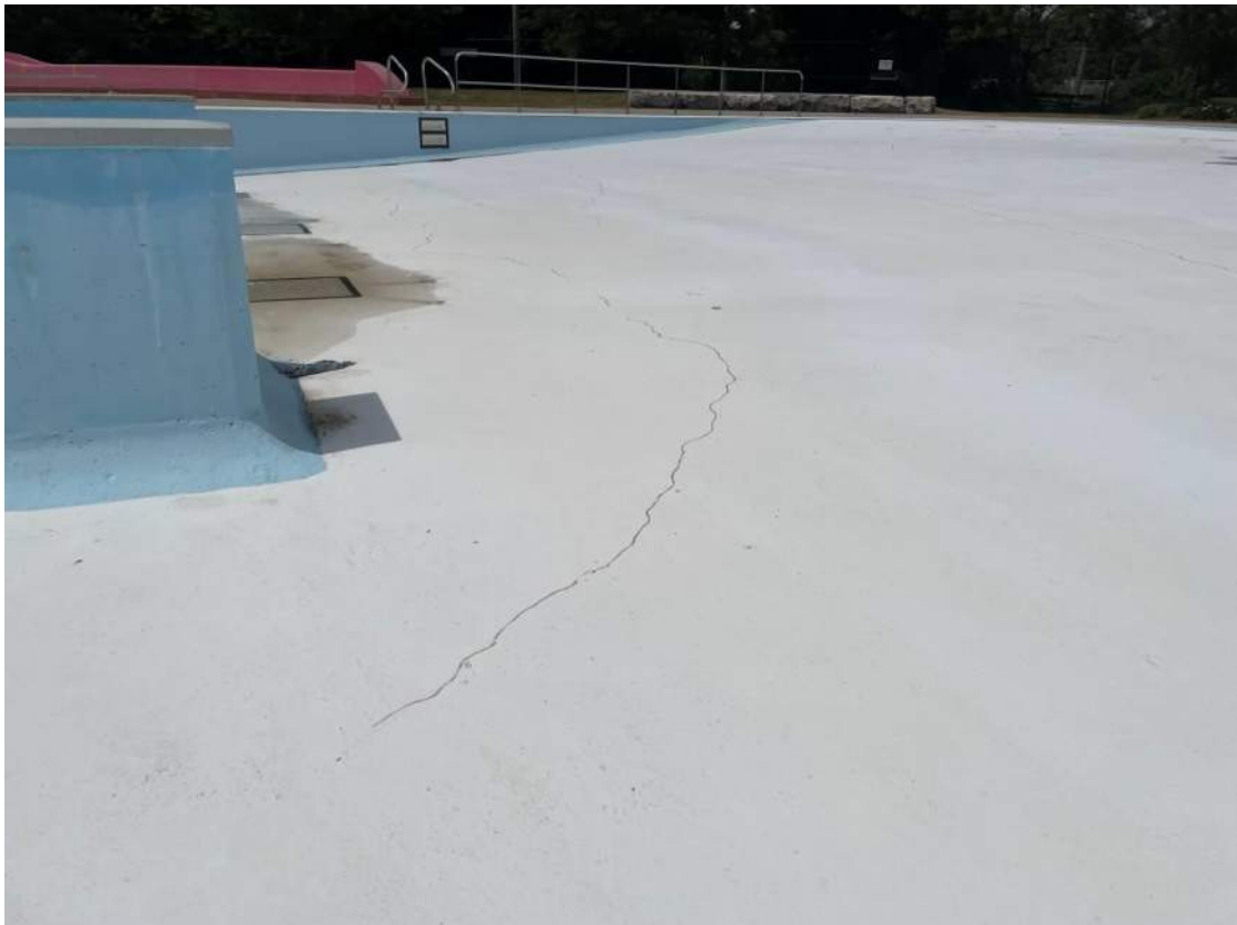
Figure 5 – Cracking within shallow end @ beach entry area
