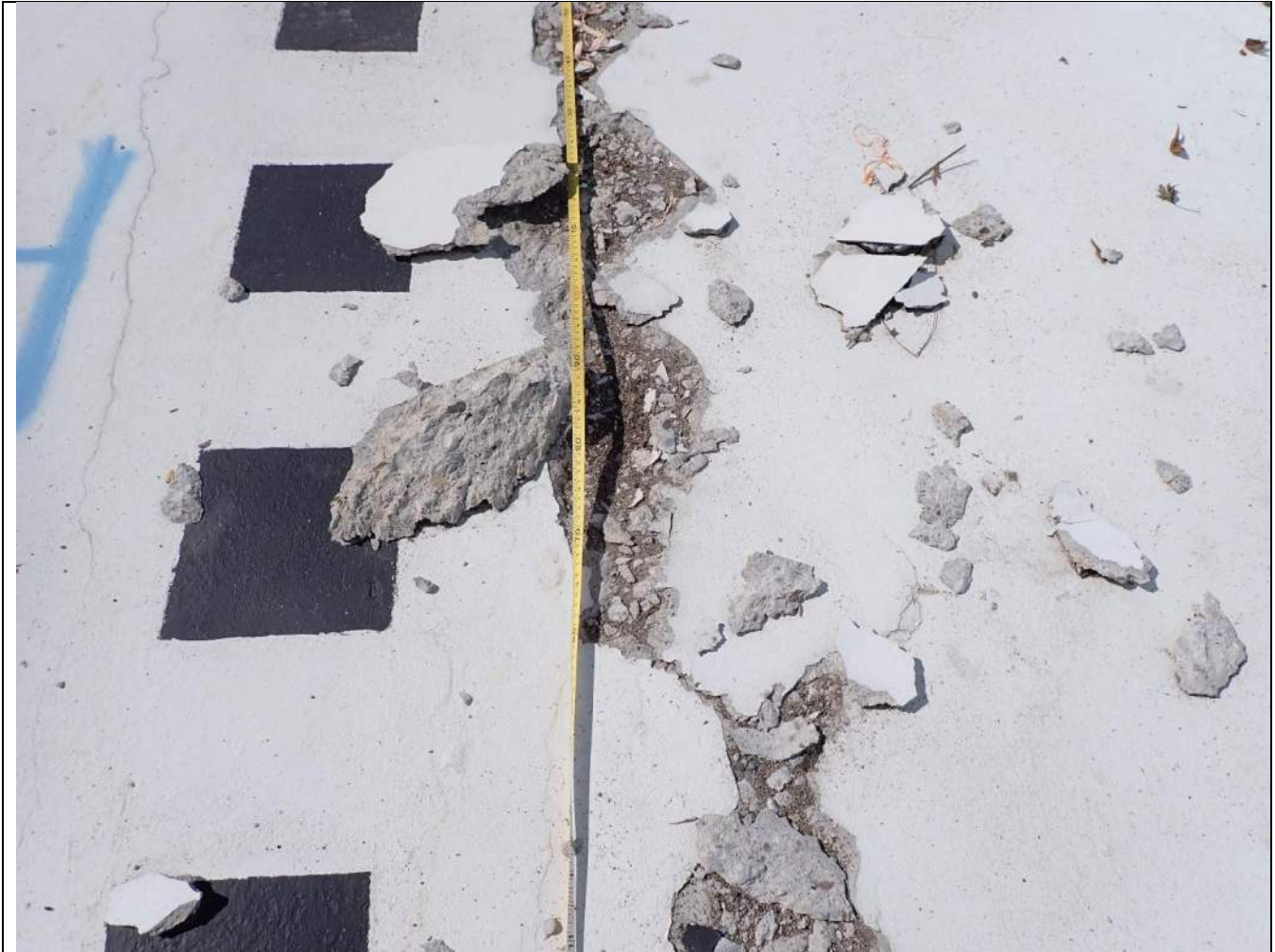
PHOTOGRAPH 10: Spalling of concrete along the crack line evident in the pool slab.
