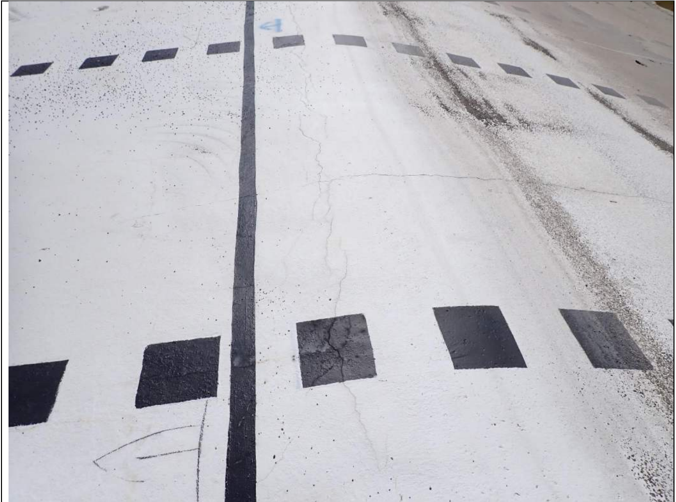
PHOTOGRAPH 9: Narrow Cracks present in the concrete forming pool floor slab.
