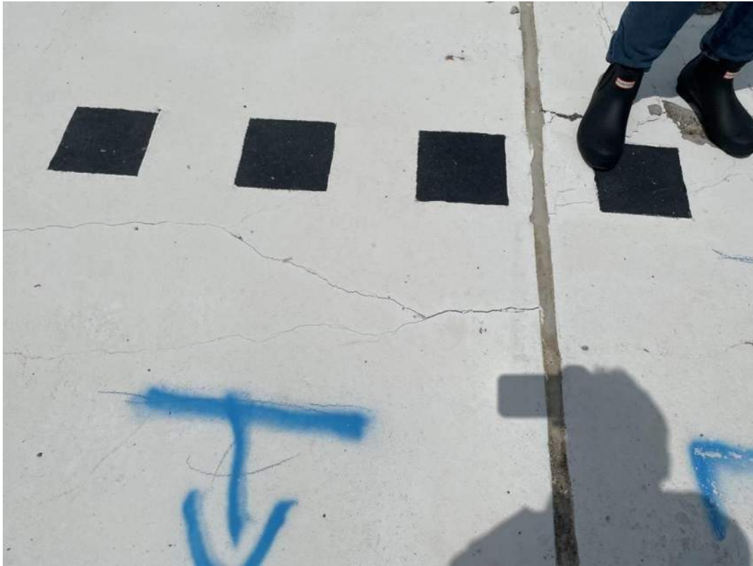
Figure 4a – Fracture in lane 1 at break point to deep area (June 2022)
