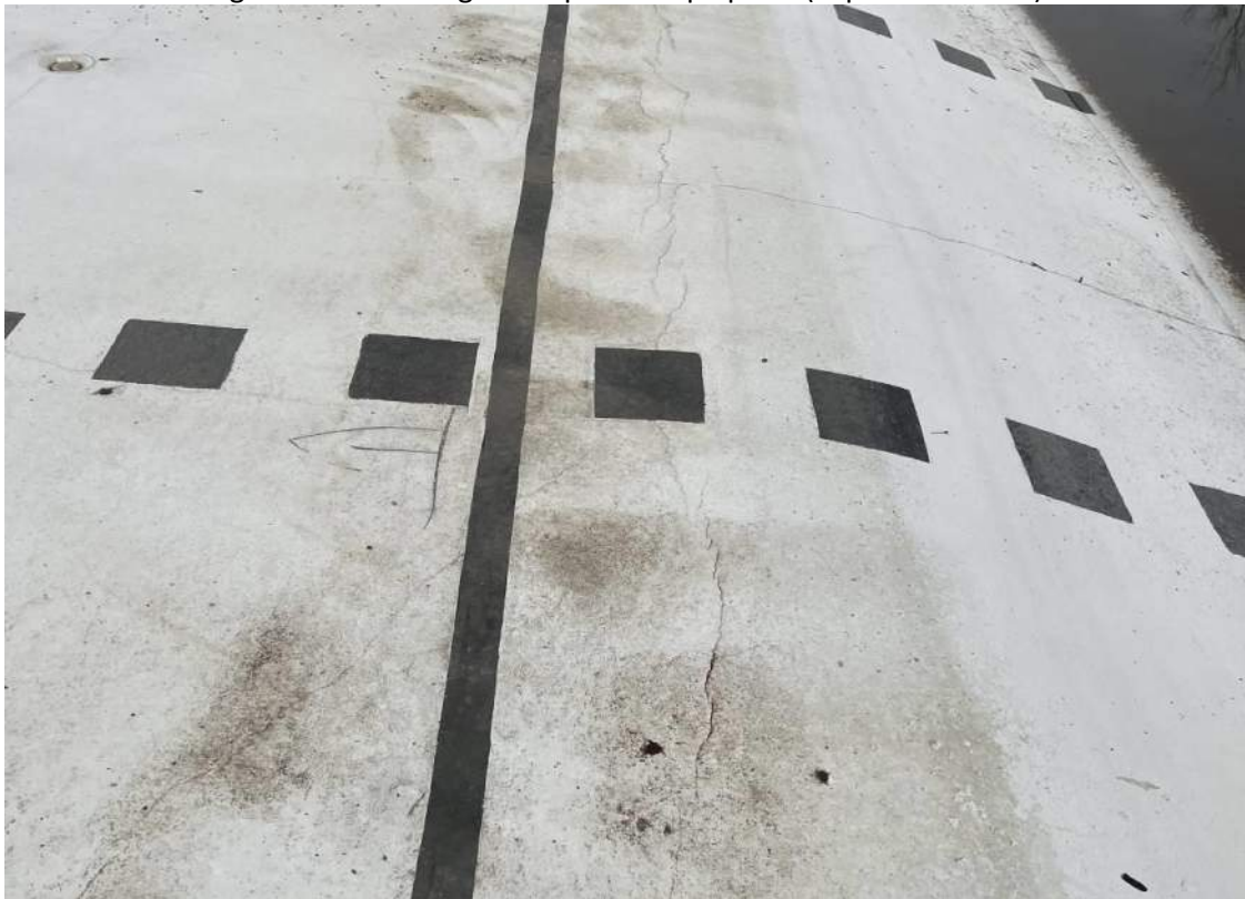
Figure 5b – Cracking at deep-end slope point (April 2023)
