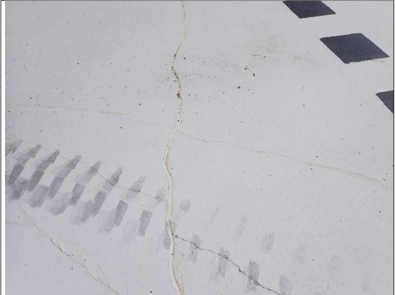
PHOTOGRAPH 7 : Large Size Cracks present in the concrete forming pool floor slab.
