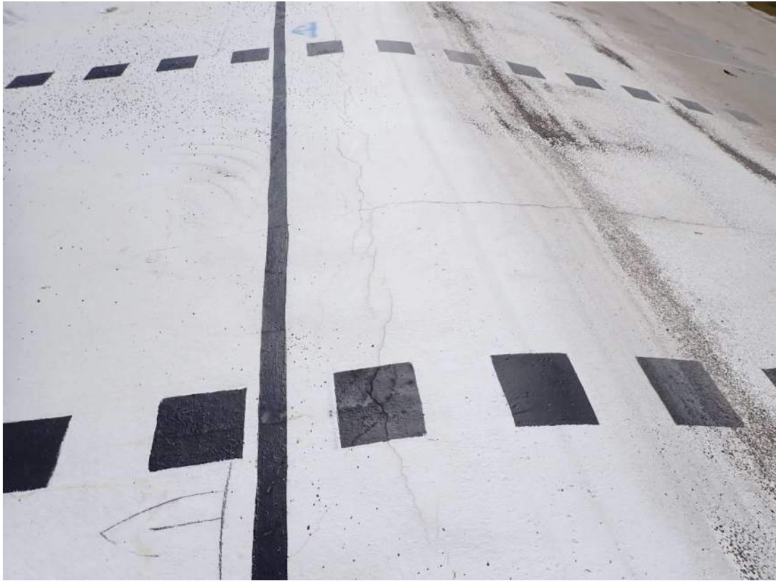
Figure 5a – Cracking at deep-end slope point (September 2022)
