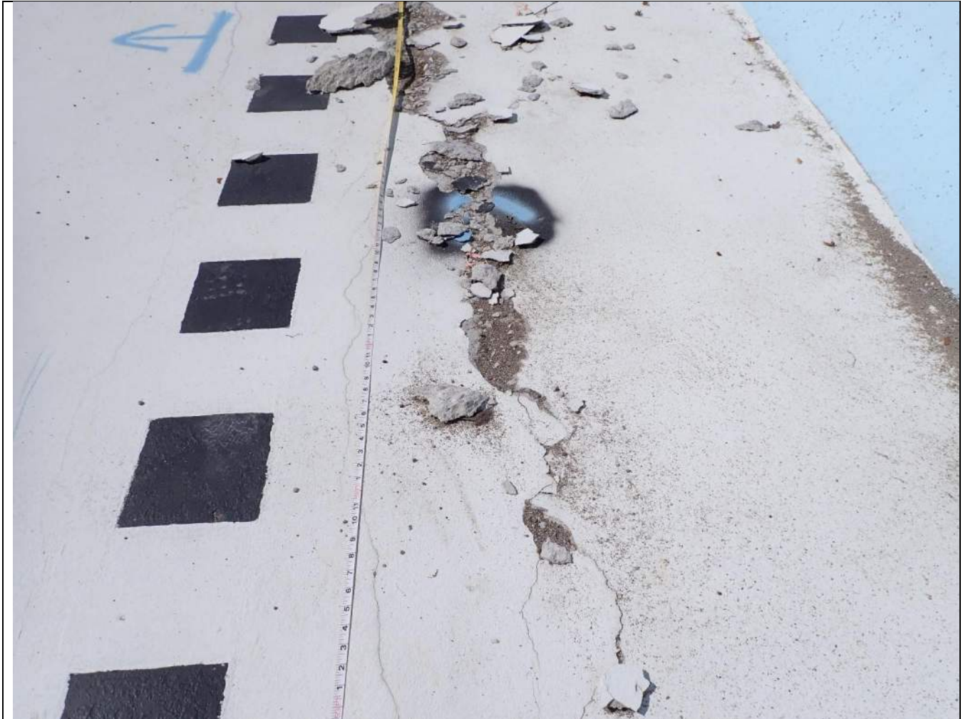
PHOTOGRAPH 12: Hydrostatic pressure evident in the form of subgrade material forced out along the crack line.
