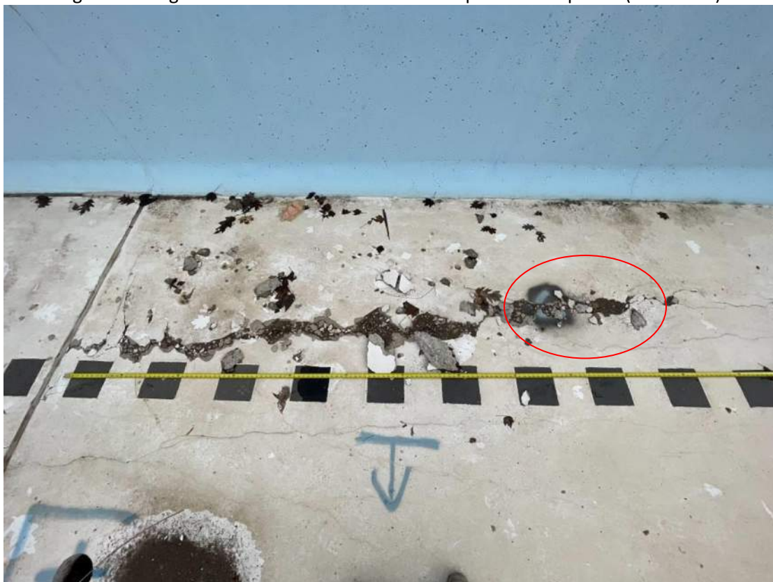
Figure 2b – Significant fracture in lane 1 at break point to deep area (April 2023)
