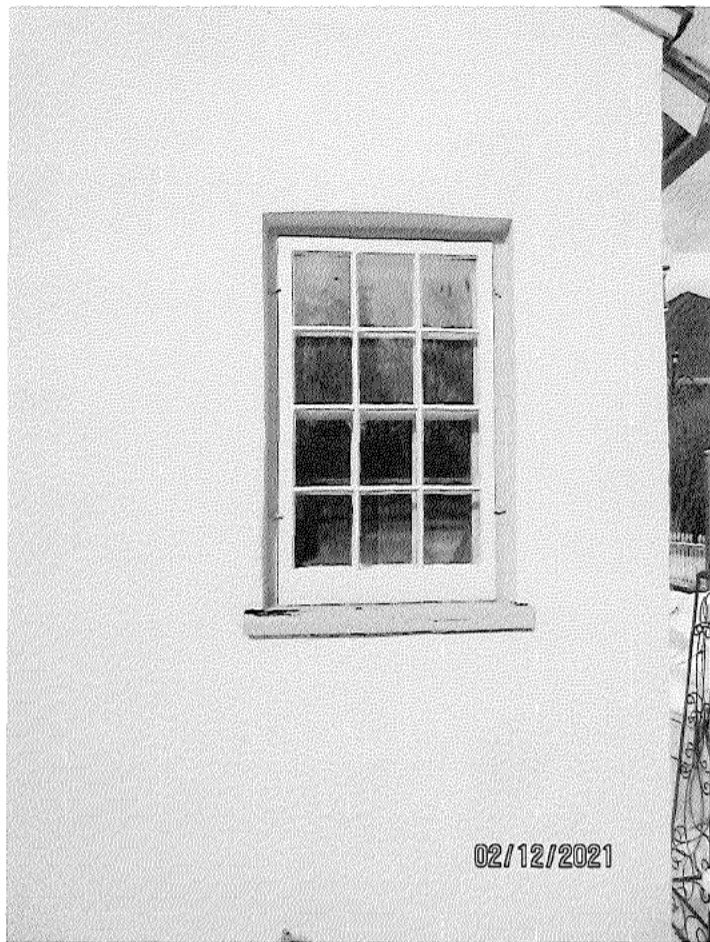
Image 29: Photograph of the six-over-six painted wood window on the south façade of the kitchen wing with a matching wood storm window and wood sill.
