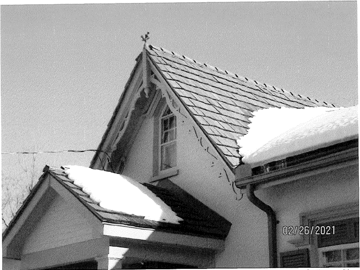
Image 18: View of the central gable dormer on the front (north) façade of Carfrae Cottage with a primitive Gothic pointed wood window and matching storm window. The decorative wood bargeboard of the central gable dormer is also shown, as well as the Scotch thistle.
