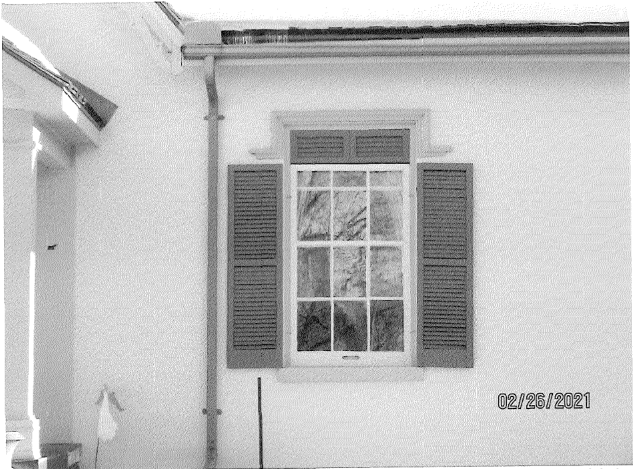
Image 17: Photograph showing the westerly front window, storm window, wood shutters, label, and sill of the front (north) façade of Carfrae Cottage.
