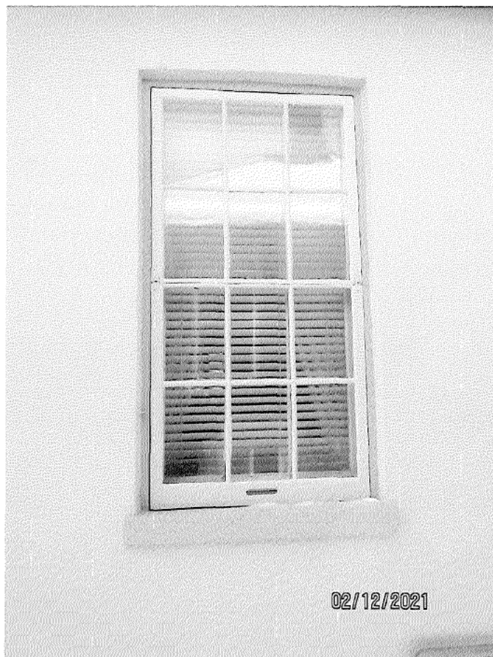
Image 34: Photograph of the six-over-six double hung painted window with matching storm window and wood sill on the east façade.
