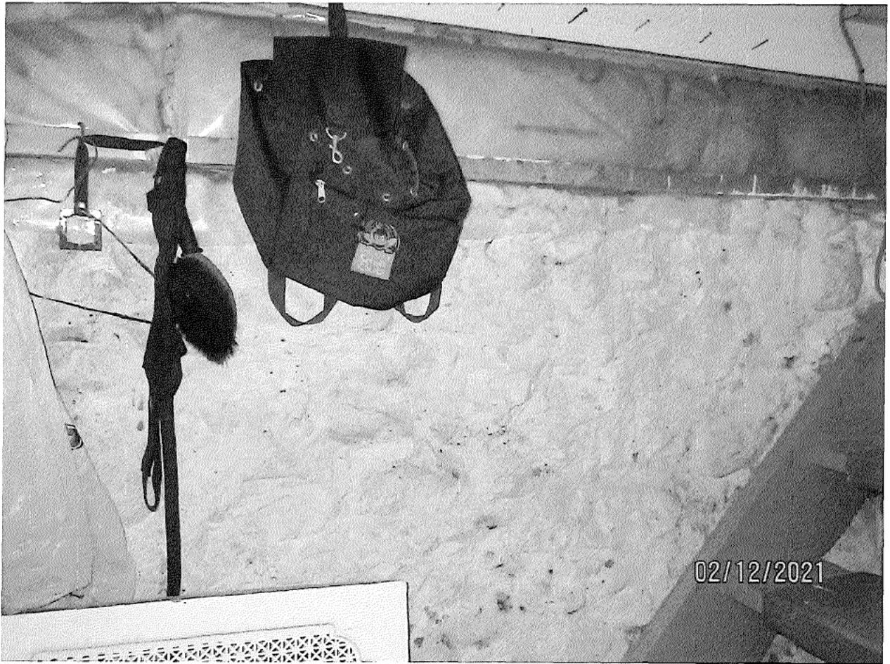
Image 7: Photograph showing an example of the rubble stone foundation construction of Carfrae Cottage, as seen in the basement.
