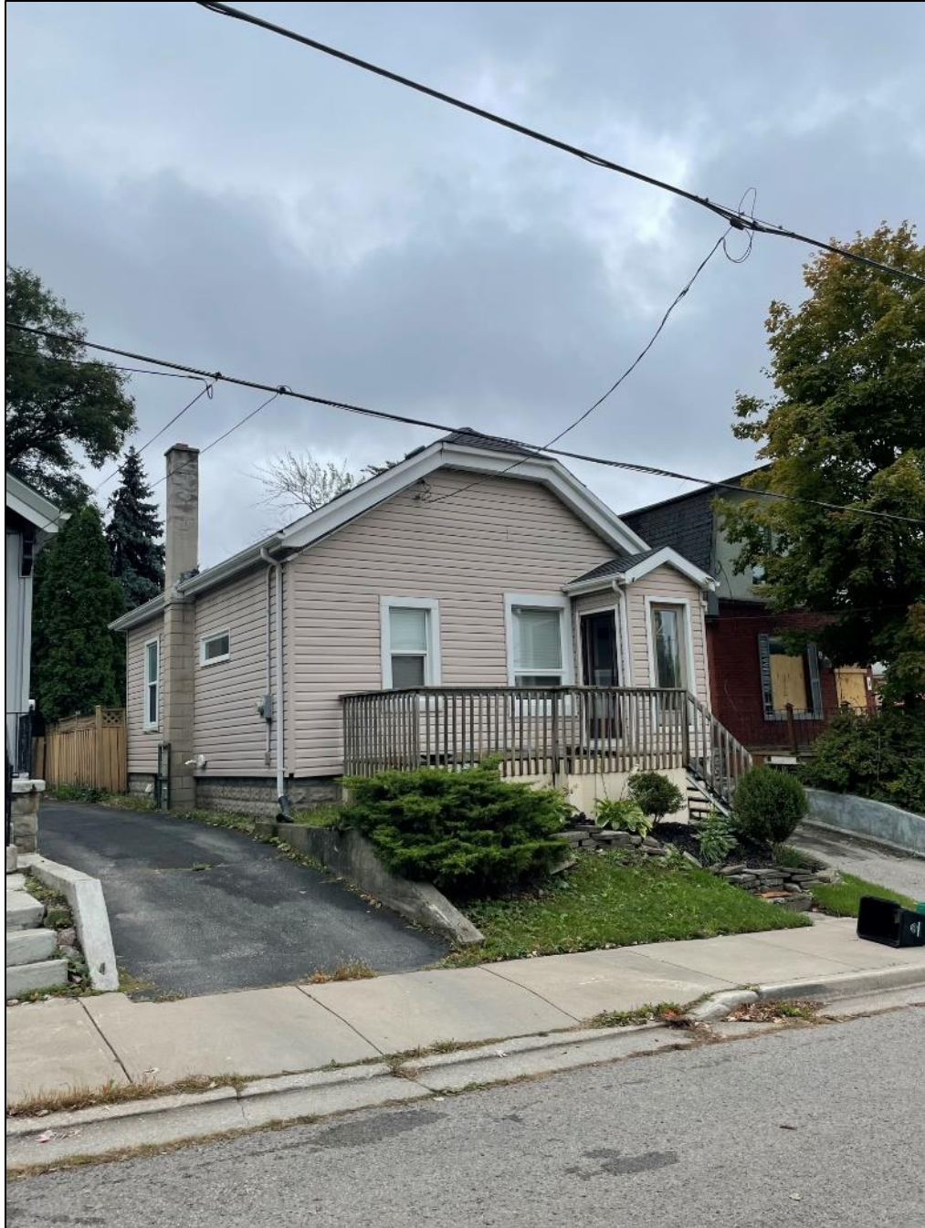
Photograph 7: View showing east side of house at 2 Kennon Place with concrete block chimney (AECOM, September 2022)
