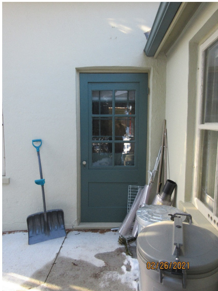
Image 24: Photograph showing the doorway, with door and storm door, on the south façade of Carfrae Cottage leading into the dining room.
