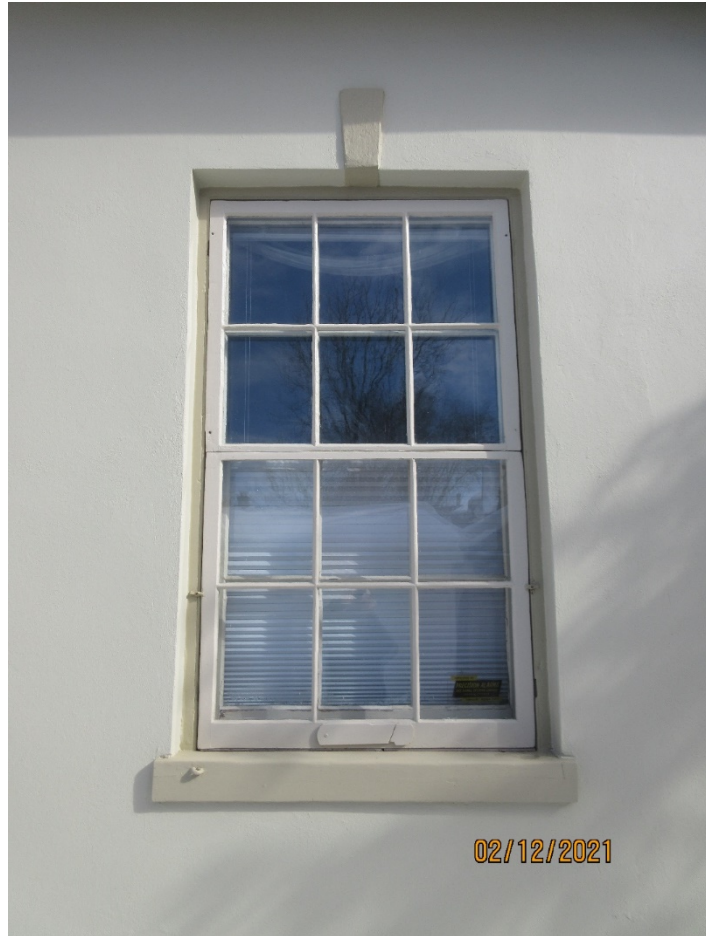
Image 21: Photograph of the painted wood six-over-six shingle hung wood window with storm windows that replicate the six-over-six fenestration. The window opening has a keystone in the parging and a wood sill.
