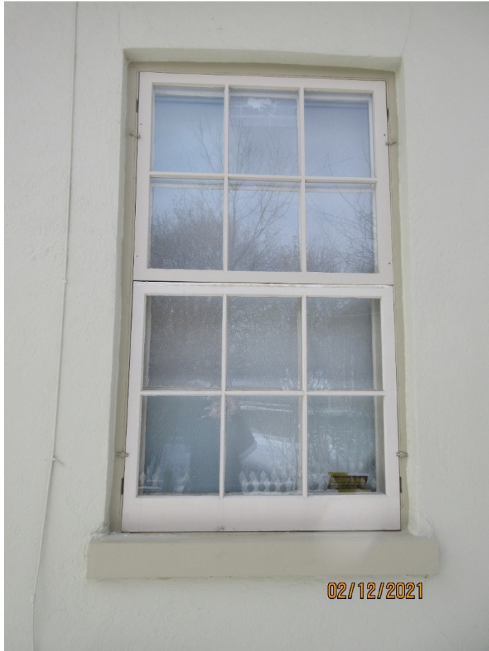
Image 33: Photograph of the six-over-six painted wood window with matching storm windows and an aluminum-clad sill.
