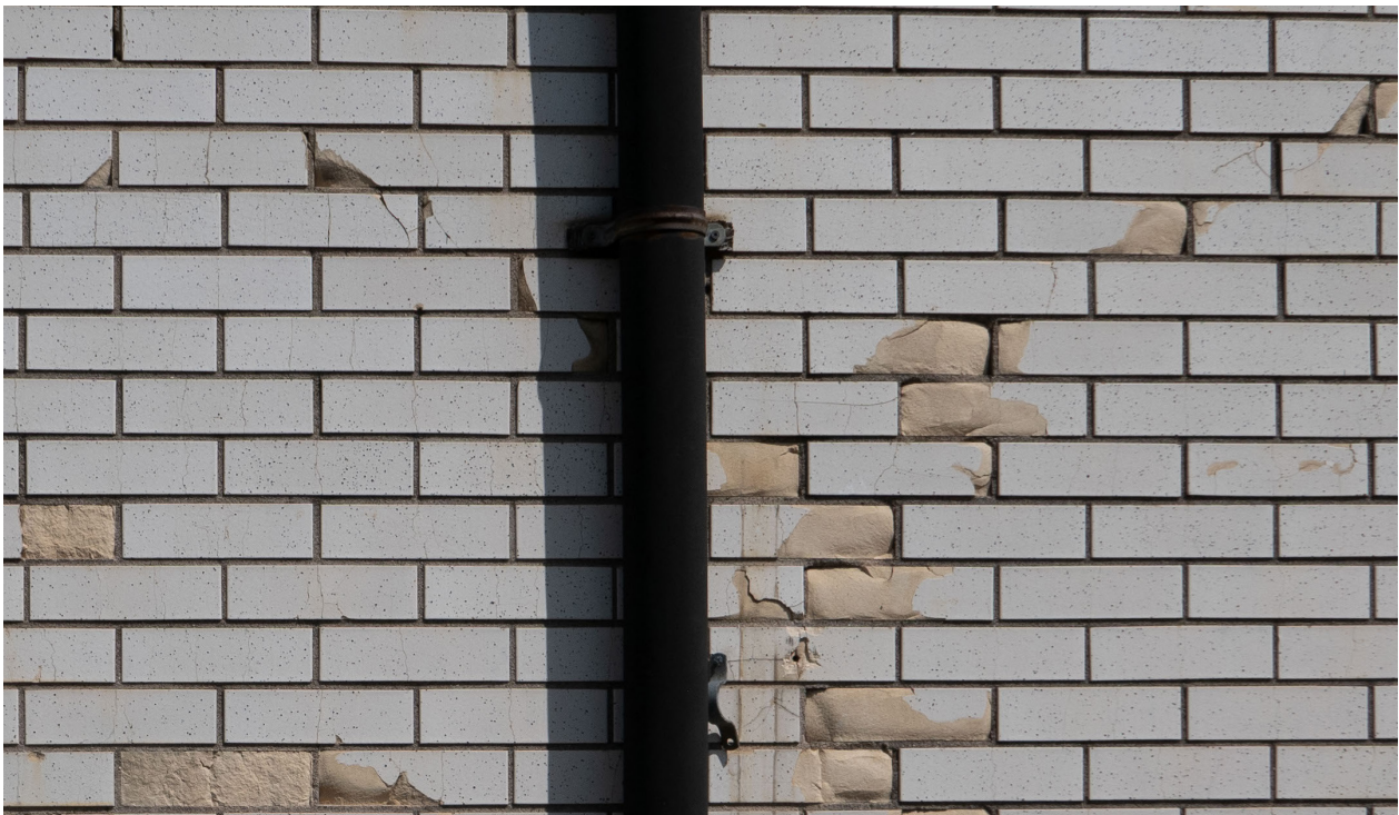
Figure 10: Detail of speckled white enamel brick on the south elevation, with damage revealing buff material beneath (CBCollective 2023).
