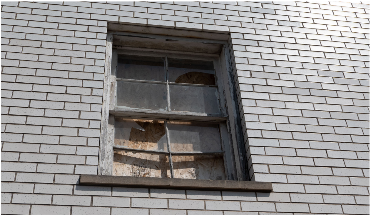
Figure 8: Remnant four-over-four wooden sash window on the south elevation, in poor condition (CBCollective 2023).
