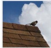
A ridge cap on a 3-tab asphalt shingle roof is composed of individual shingle "tabs" folded over the ridge and nailed partially overlapping one another
