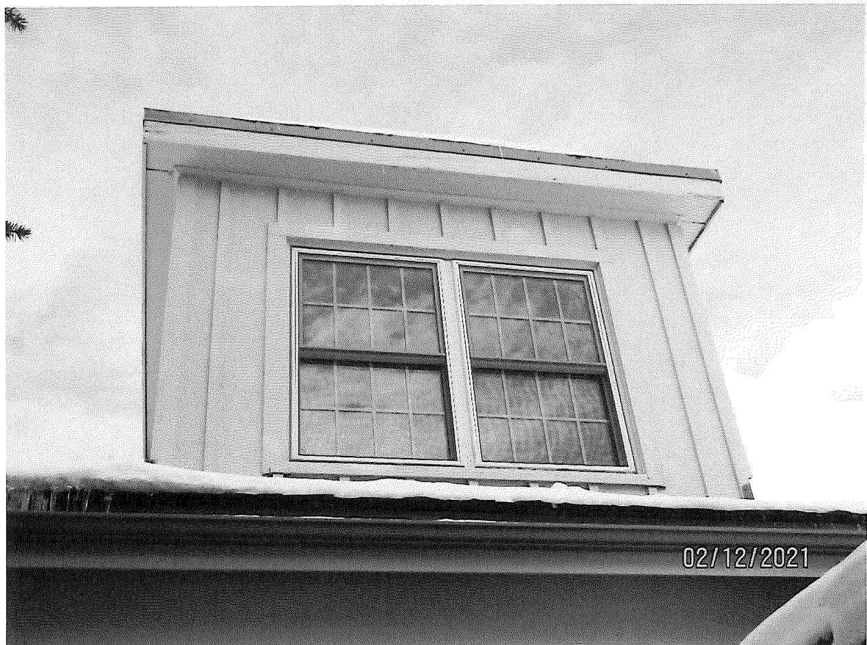
Image 28: Photograph of the shed roof dormer on the south façade of Carfrae Cottage.
