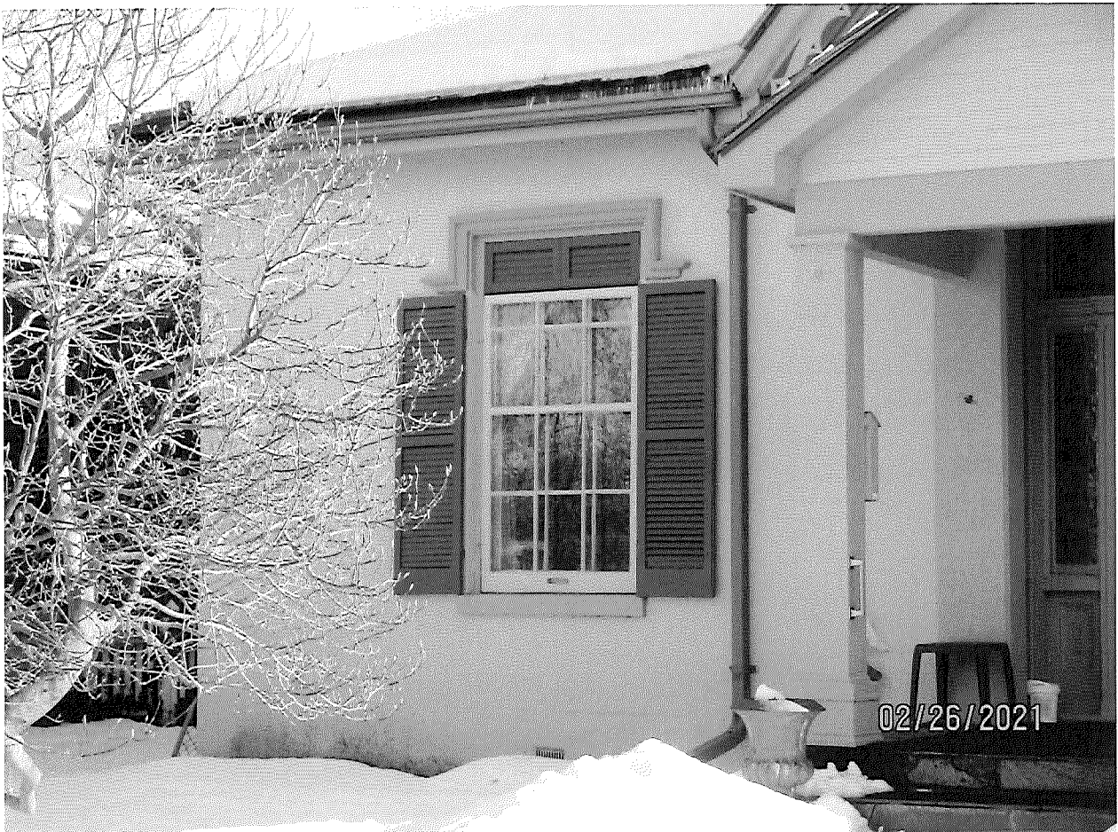
Image 16: View showing the easterly window, storm window, shutters, sill, and label on the front (north) façade of Carfrae Cottage.
