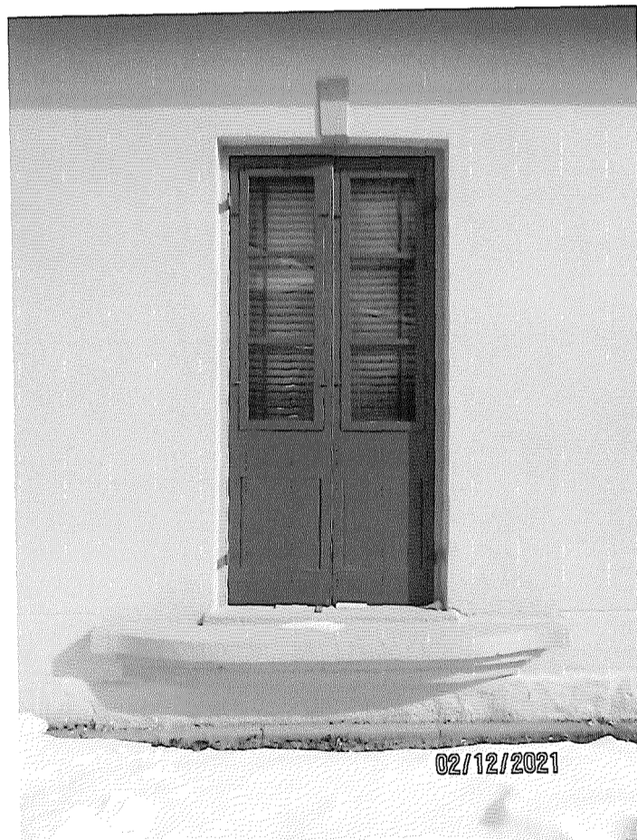
Image 20: Photograph of the painted wood French doors and painted wood storm doors in the northerly opening of the west façade, which retains its cast sill as an indication of the former verandah of Carfrae Cottage. The doorway has a keystone in the parging.
