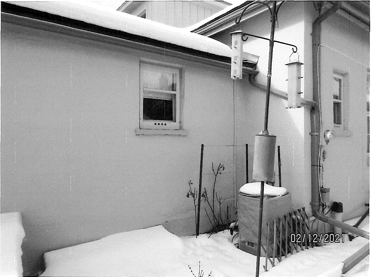
Image 31: Showing the junction of the kitchen wing and the house along the easterly façade of Carfrae Cottage.
