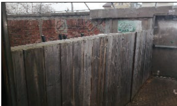
Figure 27: View of interior of west side of north elevation from interior of Joe Kool's restaurant looking north-west (Source: MHBC, 2020).
