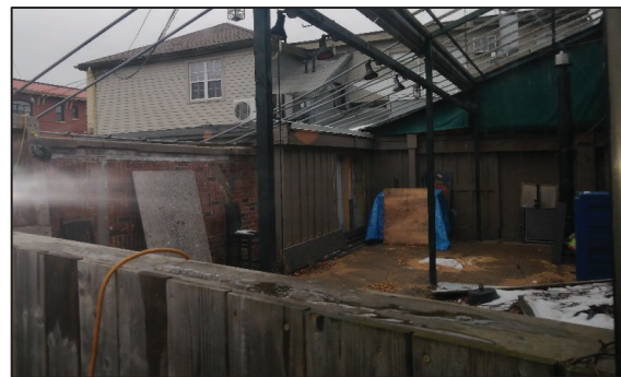
Figure 28: View of interior of east side of north elevation from the interior of restaurant looking north-east (Source: MHBC, 2020).
