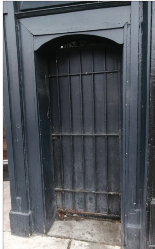
Figure 39: View of door opening/ access that leads to alleyway to brick ancillary structure to the rear of 595 Richmond Street (Source: MHBC, 2020).
