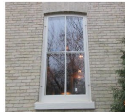
8. Exceptionally large (7 feet in height), two-over-two wood windows, with wood storm windows, on the main floor
