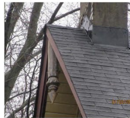
4. Heavy finial and drop in the north gable
