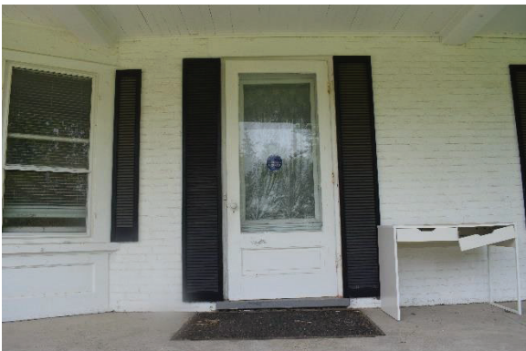
Plate 22: Main entrance door, looking south
