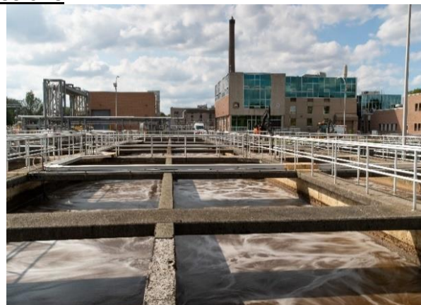
Greenway Wastewater Treatment Plant
