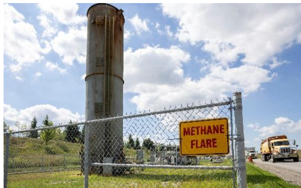
The methane flare stack at the W12A Landfill
