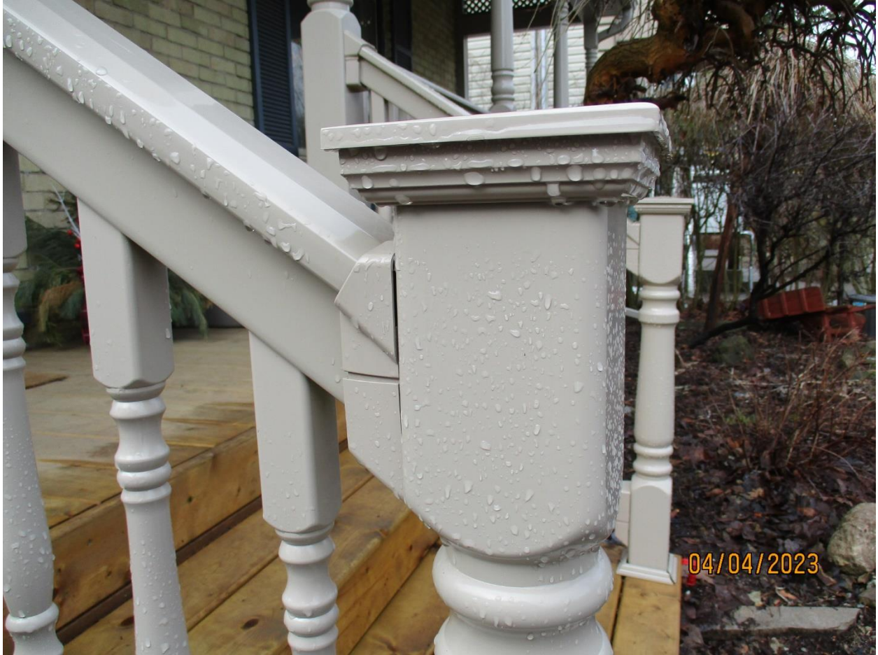
Image 6: Photograph showing detail of the vinyl (plastic) porch materials used for the replacement of the porch at 27 Bruce Street within the Wortley Village-Old South Heritage Conservation District.
