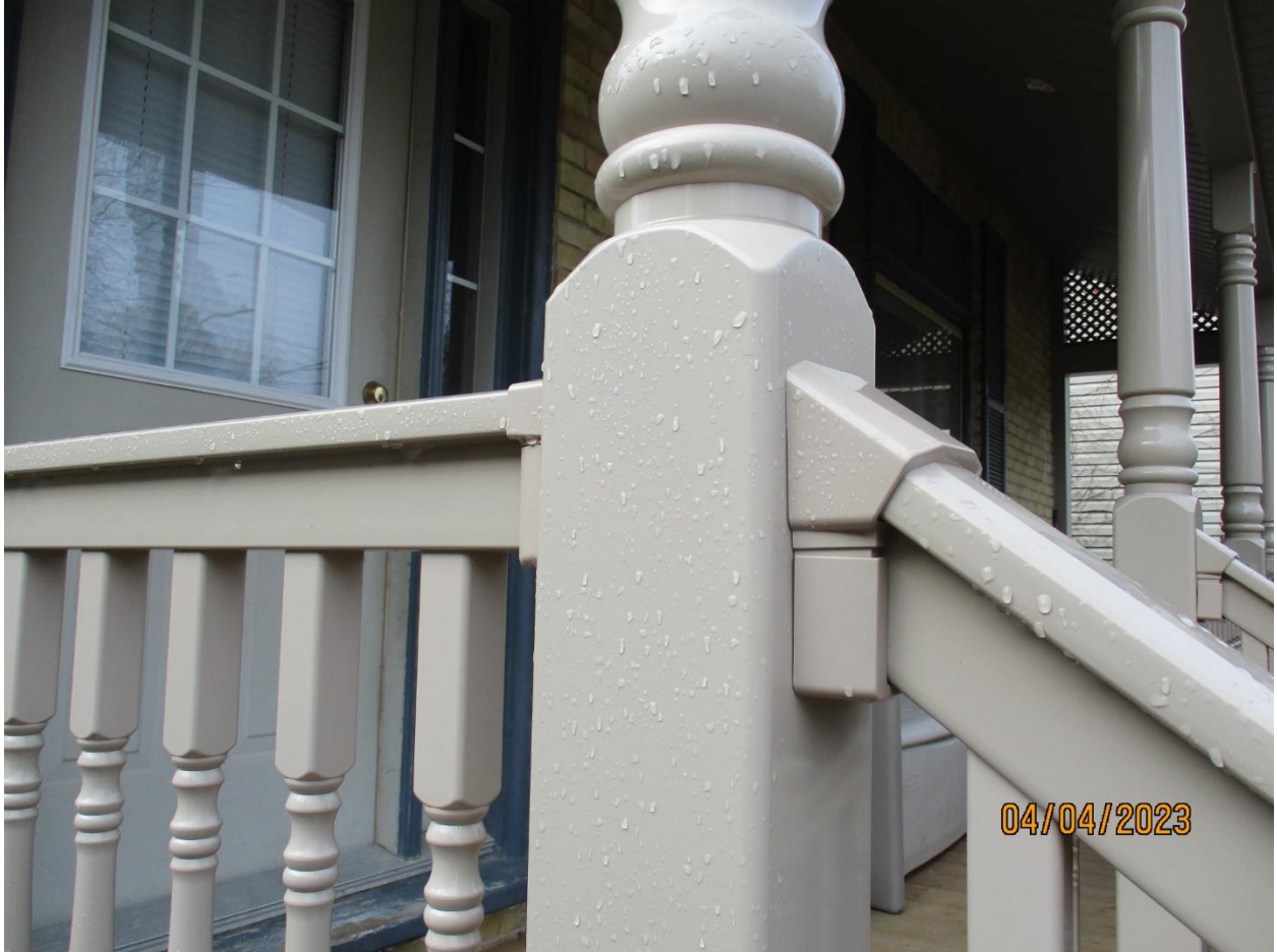
Image 8: Photograph showing detail of the vinyl (plastic) porch materials used for the replacement of the porch at 27 Bruce Street within the Wortley Village-Old South Heritage Conservation District.
