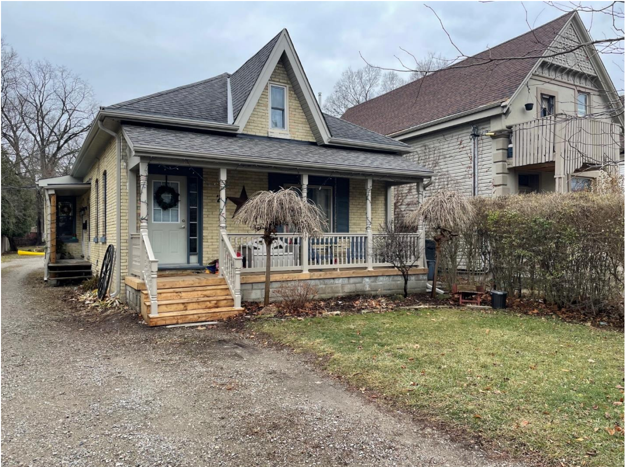
Image 2: Photograph submitted with the Heritage Alteration Permit application showing the porch with vinyl-clad (plastic) posts and vinyl railings, with pressure-treated decking.
