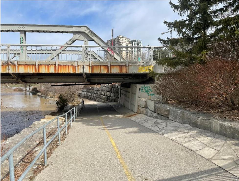
Photograph 20: View of the east end abutment and TVP below bridge (AECOM, April 2023)
