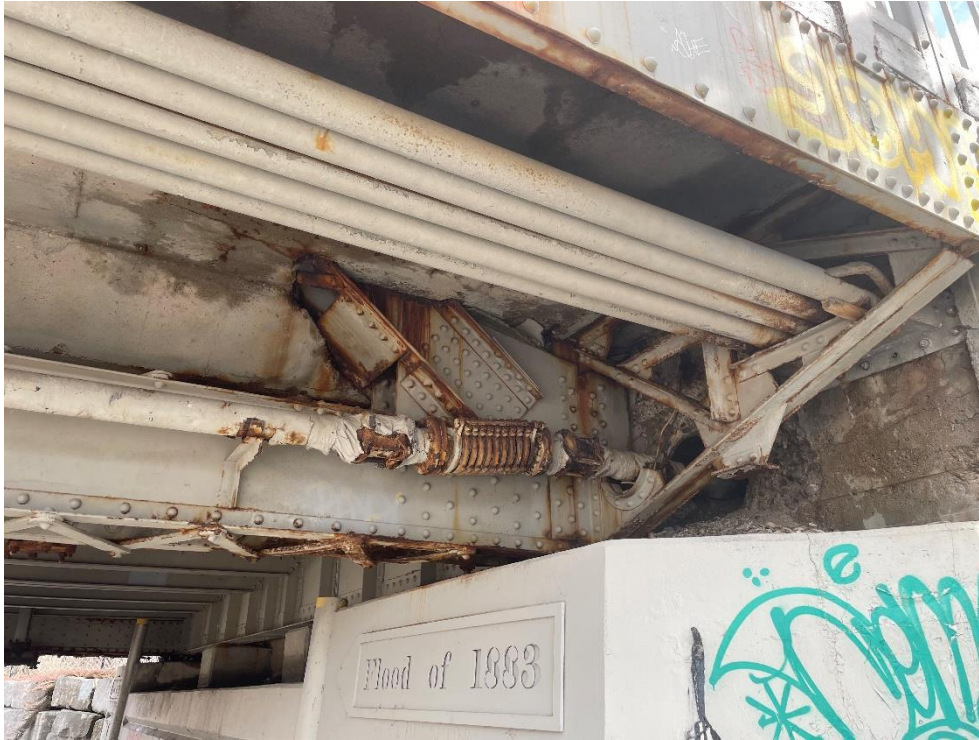
Photograph 22: View of underside of bridge at the east abutment with conduits (AECOM, April 2023)
