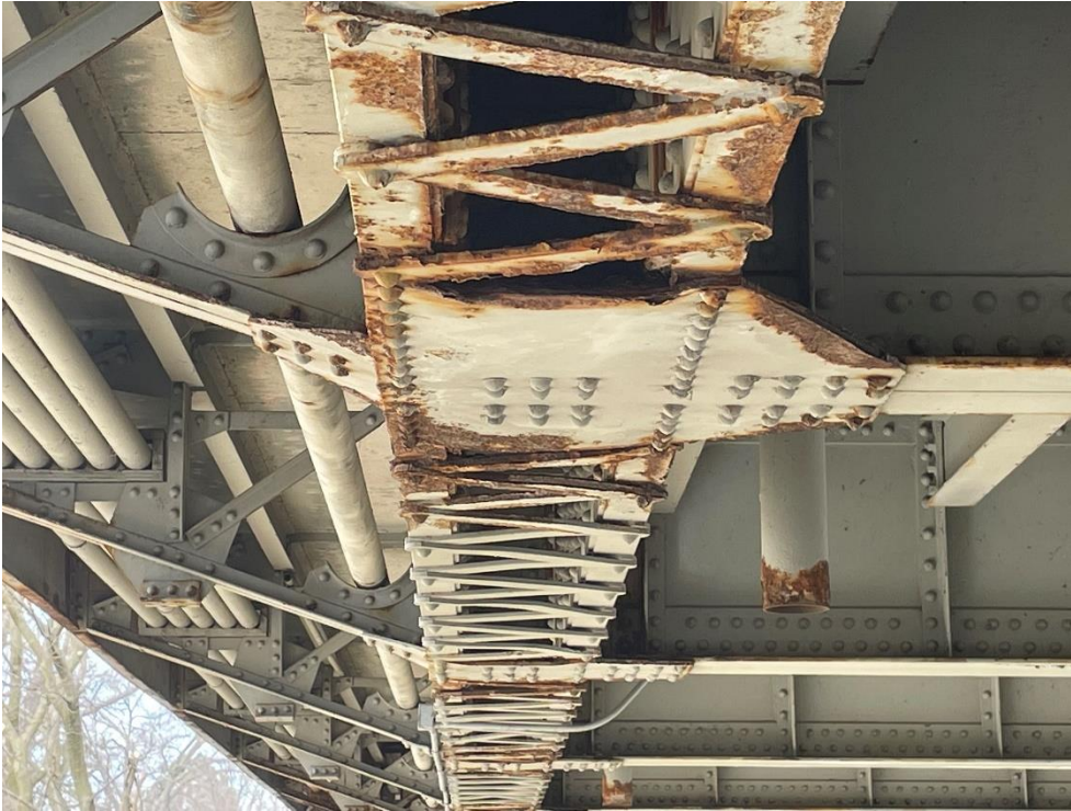
Photograph 26: View of V-lacing on the bottom chord with gusset plates (AECOM, April 2023)
