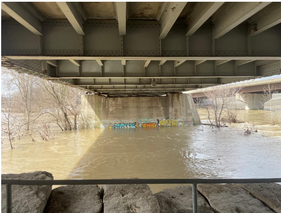
Photograph 23: View of the east pier from the underside of the east end of the bridge (AECOM, April 2023)
