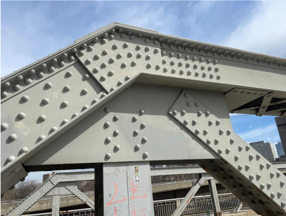
Photograph 12: Top chord connections, including steel gusset plates, as viewed from the south sidewalk (AECOM April 2023)
