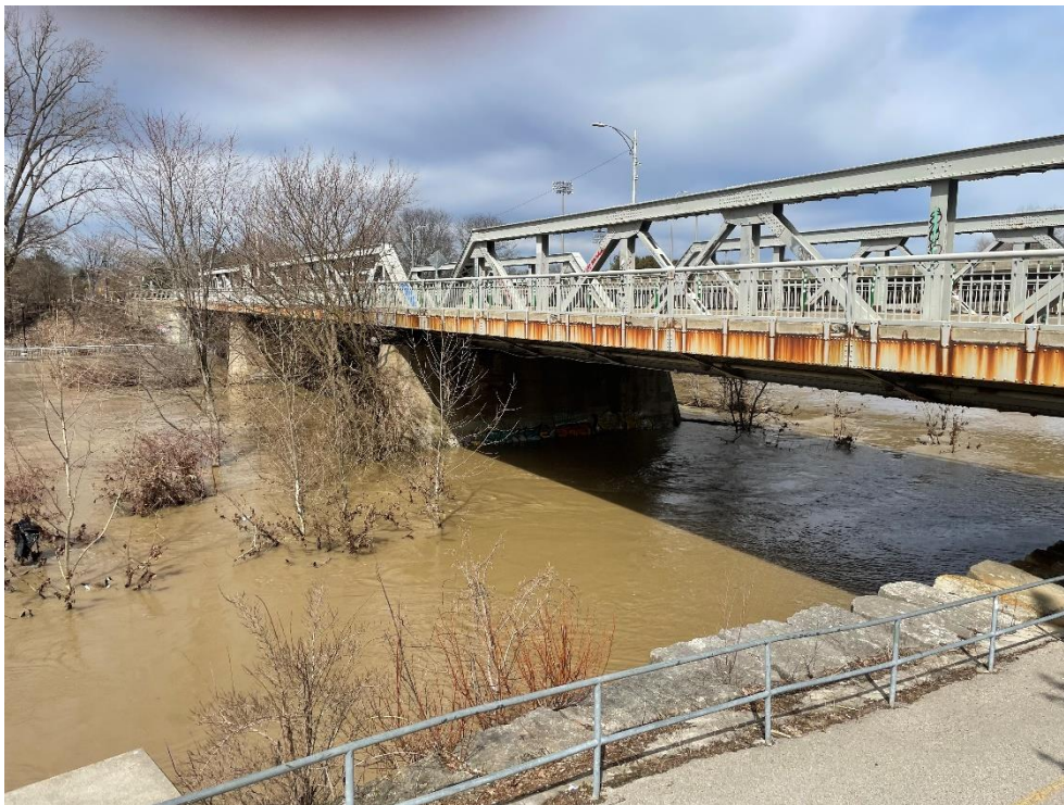
Photograph 19: Oblique view of the south elevation from the southeast quadrant and piers (AECOM, April 2023)
