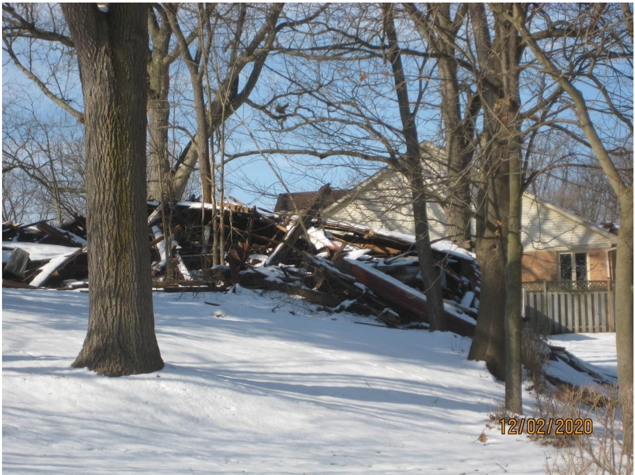
Image 10: Photograph showing the property in February 2020, following the unapproved demolition of the accessory building.
