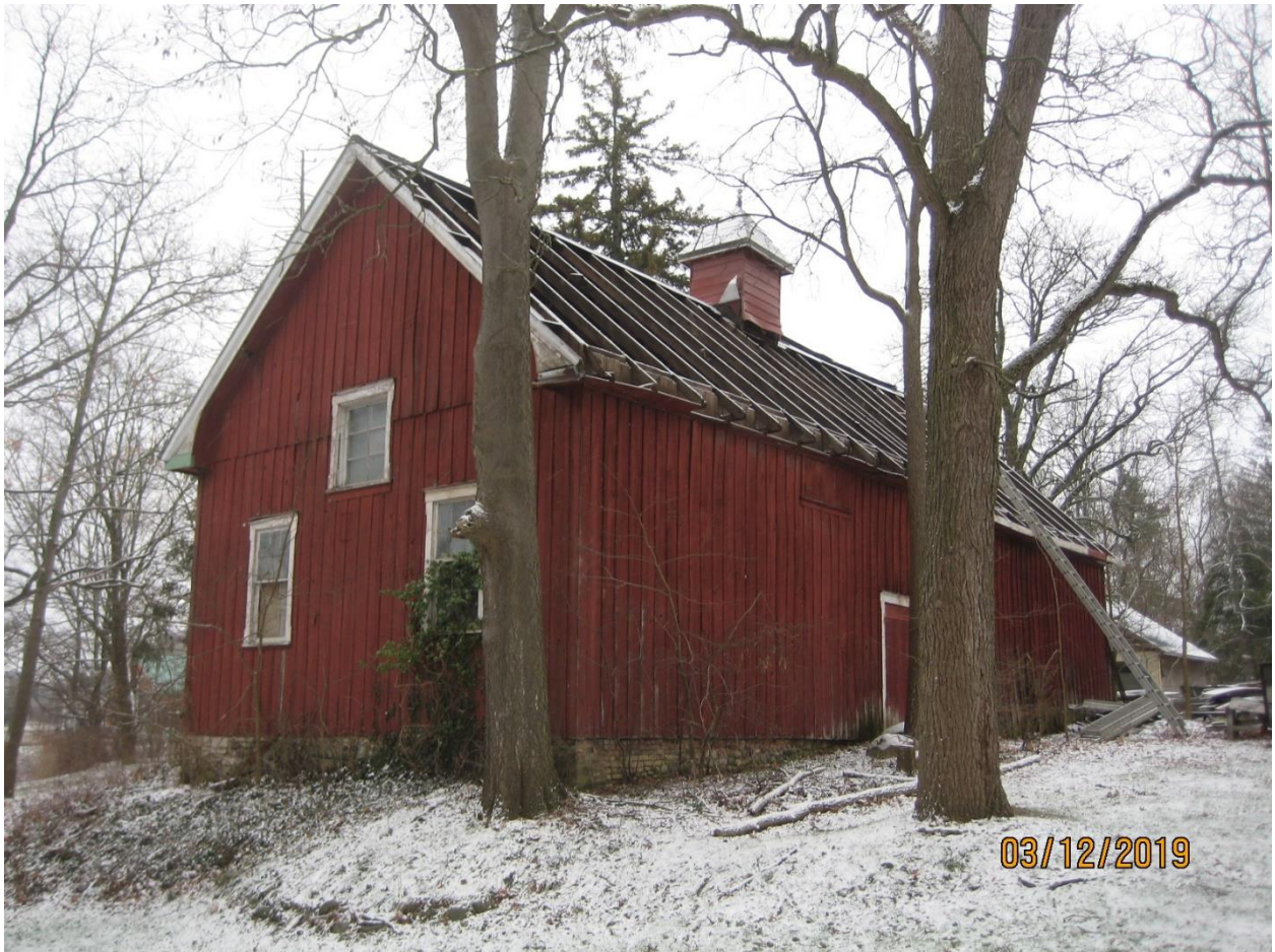
Image 5: Photograph of the west side of the accessory building, showing the removed roof sheathing, December 3, 2019.
