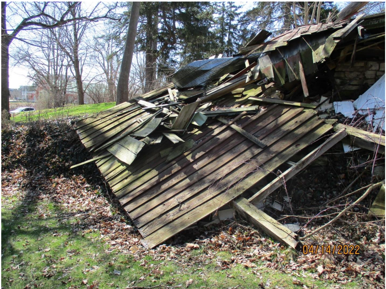
Image 14: Photograph showing debris from the former accessory building, shown in April 2022. Note, a portion of the rubble stone foundation can be seen buried under the debris at right. A portion of the cherry board-and-batten exterior cladding can be seen at centre.
