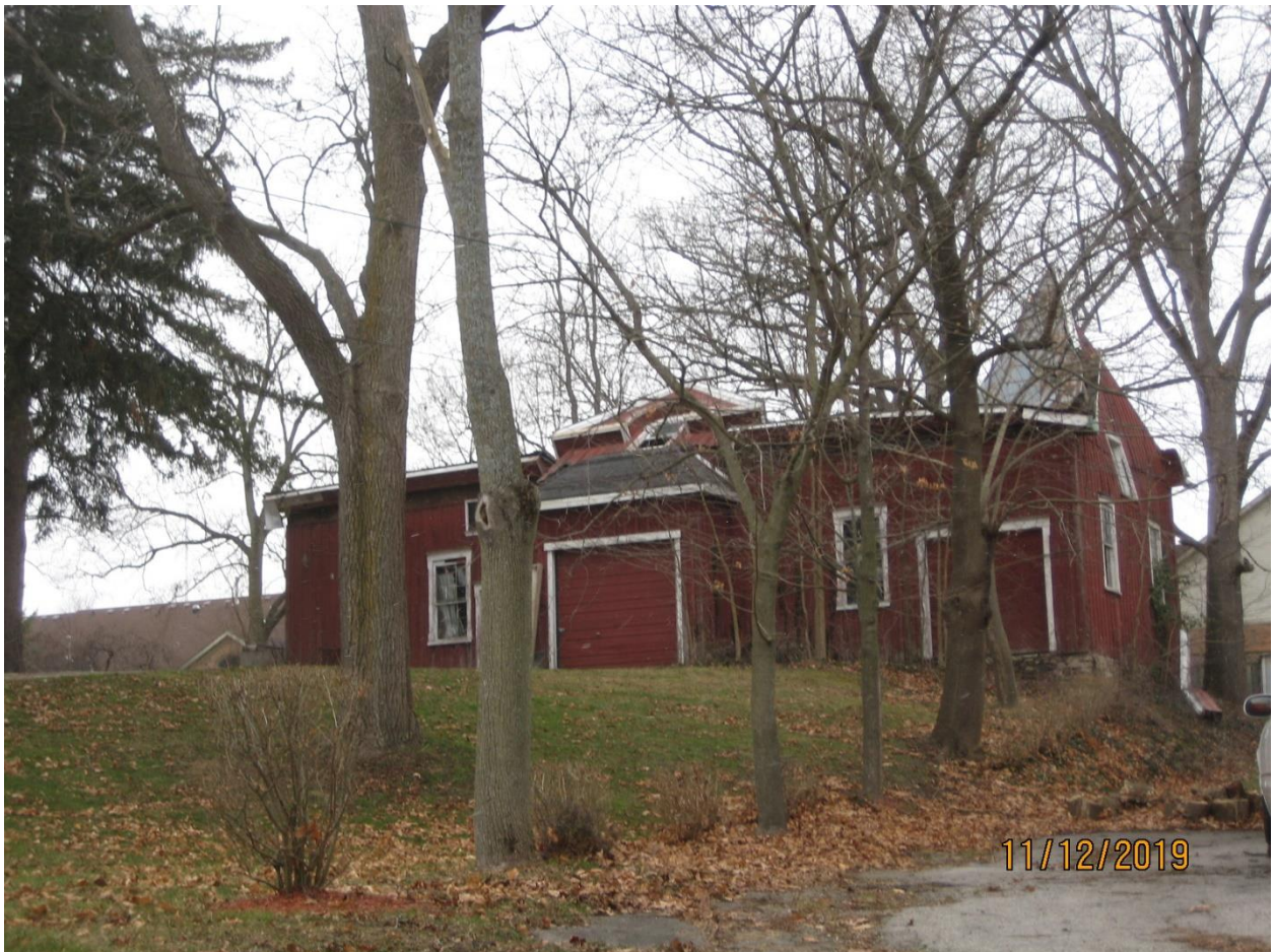
Image 8: Photograph showing the east side of the accessory building as viewed from Halls Mill Road, showing the collapse of the roof framing, December 11, 2019.
