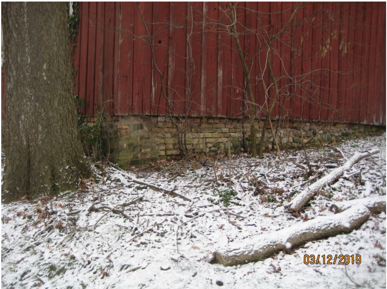
Image 6: Photograph of the foundation on the west side of the accessory building showing a mix of buff brick and field stone materials, December 3, 2019.
