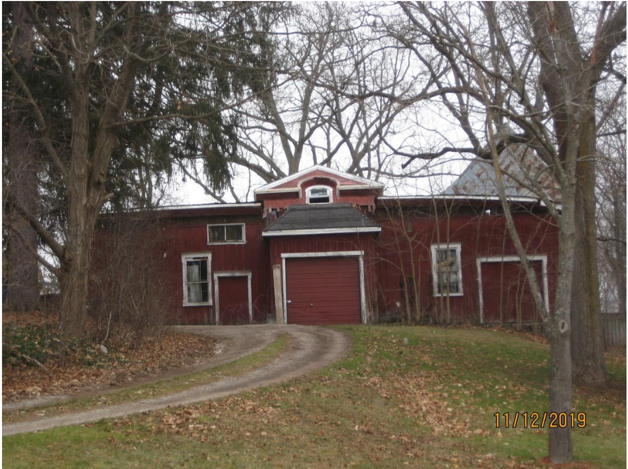
Image 7: Photograph showing the east side of the accessory building as viewed from Halls Mill Road, showing the collapse of the roof framing, December 11, 2019.
