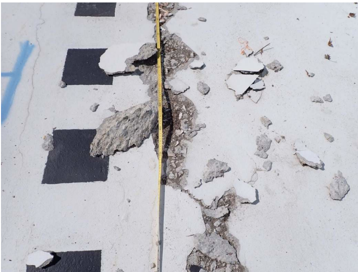
Photo 5/6 - Indication of Pool Movement
