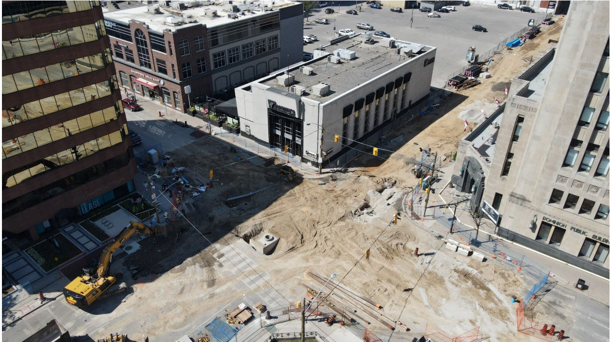
Above: Aerial view the Downtown Loop Phase 2 construction site at the Queens Avenue and Richmond Street intersection.
