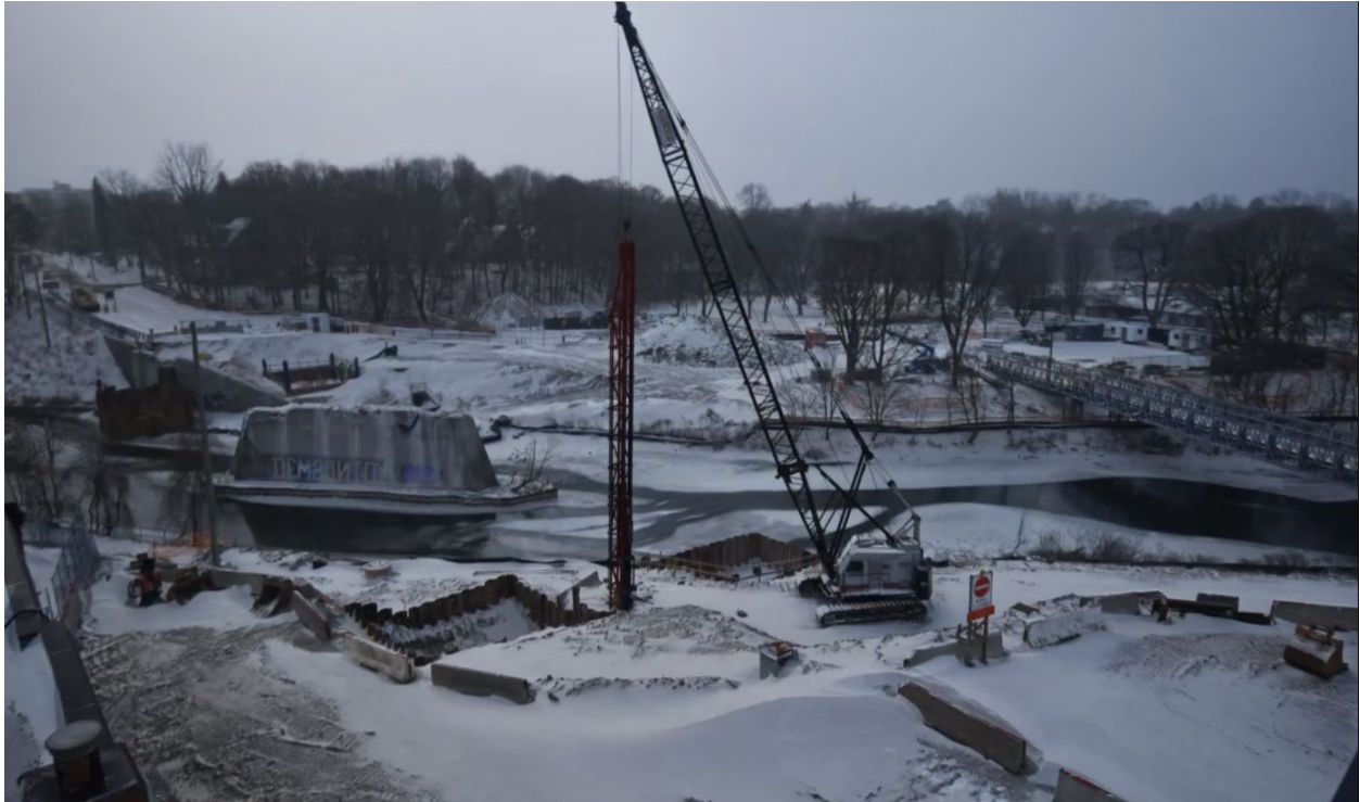
Above: Aerial view of construction works at the Victoria Bridge on Ridout Street North.
