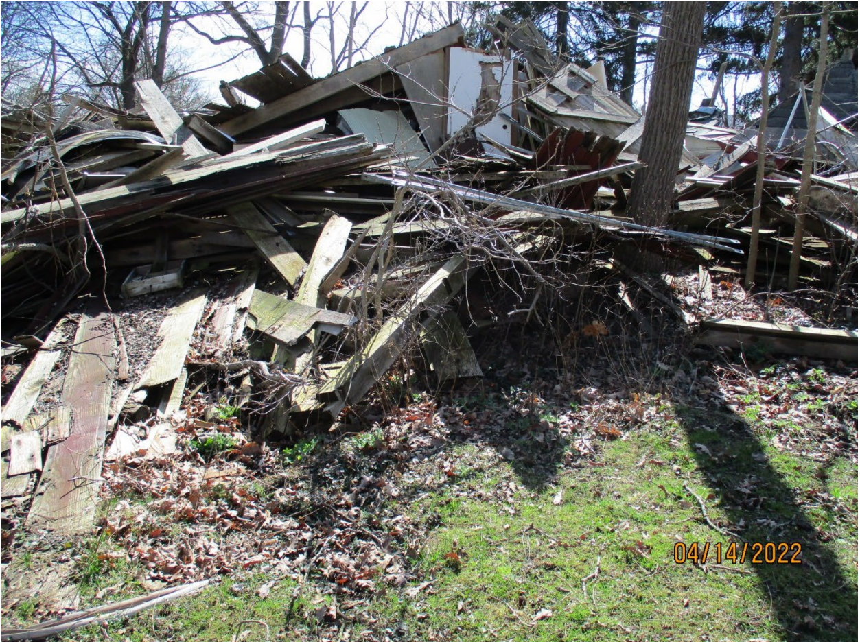
Image 11: Photograph of the debris from the former accessory building, shown in April 2022.
