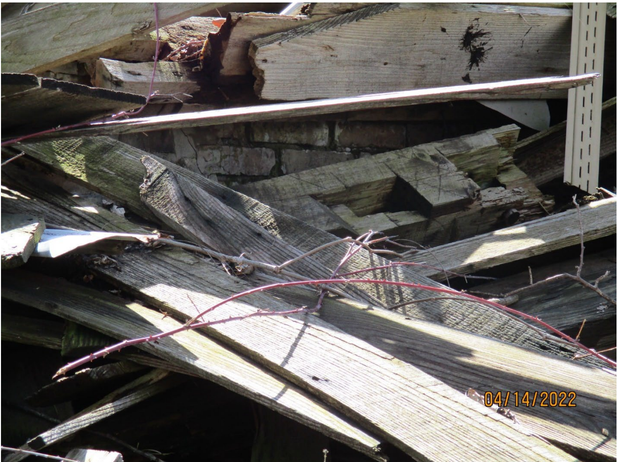
Image 12: Photograph showing debris from the former accessory building, shown in April 2022. Note, a portion of the buff brick foundation can be seen buried under the debris.
