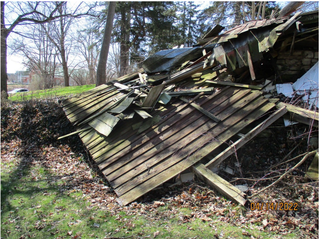
Image 14: Photograph showing debris from the former accessory building, shown in April 2022. Note, a portion of the rubble stone foundation can be seen buried under the debris at right. A portion of the cherry board-and-batten exterior cladding can be seen at centre.
