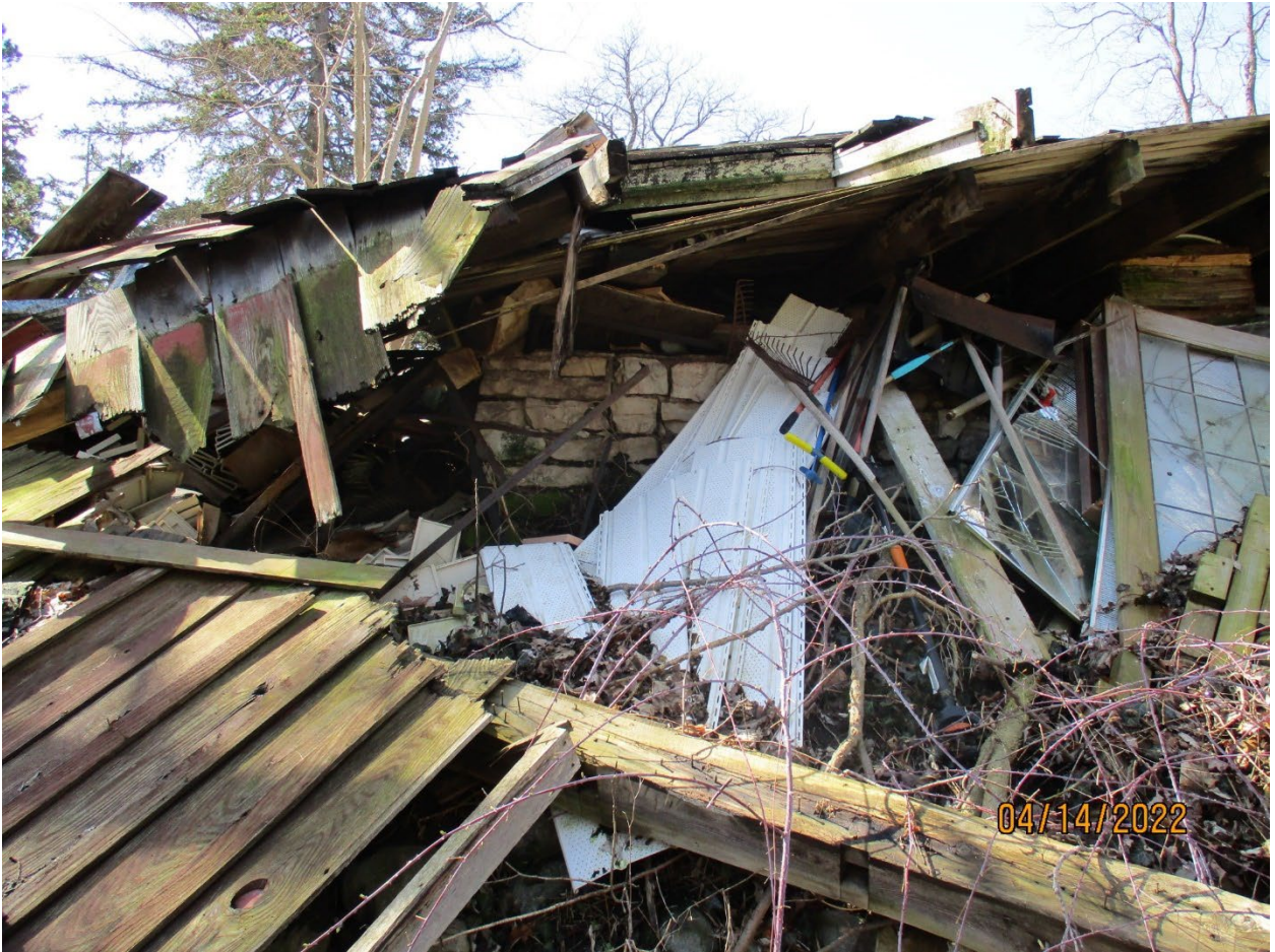
Image 13: Photograph showing debris from the former accessory building, shown in April 2022. Note, a portion of the rubble stone foundation can be seen buried under the debris.
