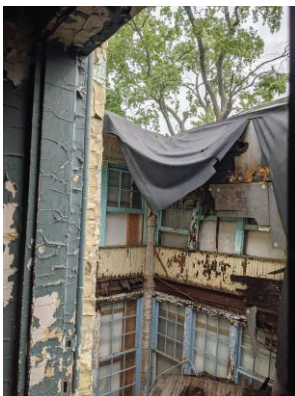
Photo 14: East porch collapse in June 2021
