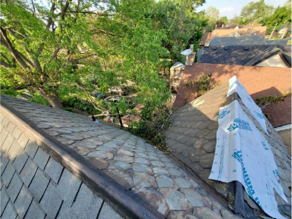
Image 11: Photograph submitted as a part of an inspection report showing extent of damage to the slate roof.
