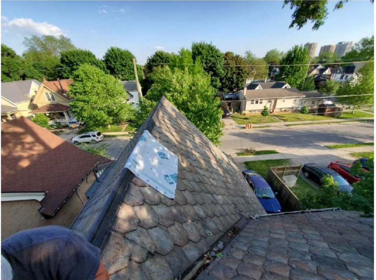
Image 9: Photograph submitted as a part of an inspection report showing extent of damage to the slate roof.
