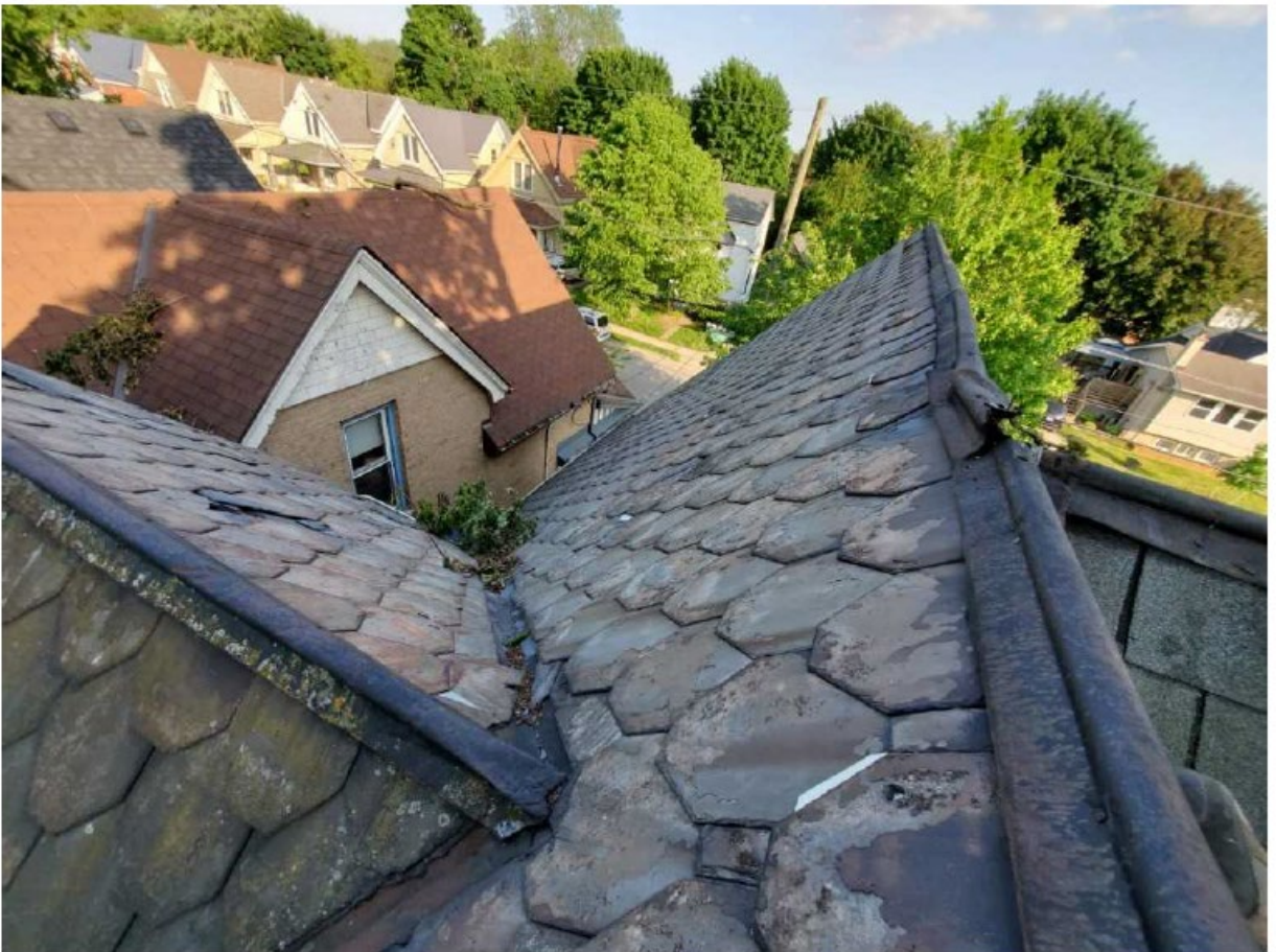
Image 10: Photograph submitted as a part of an inspection report showing extent of damage to the slate roof.
