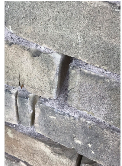
Signs of mortar failure. Photo by: a+LiNK Architecture Inc., 2020
