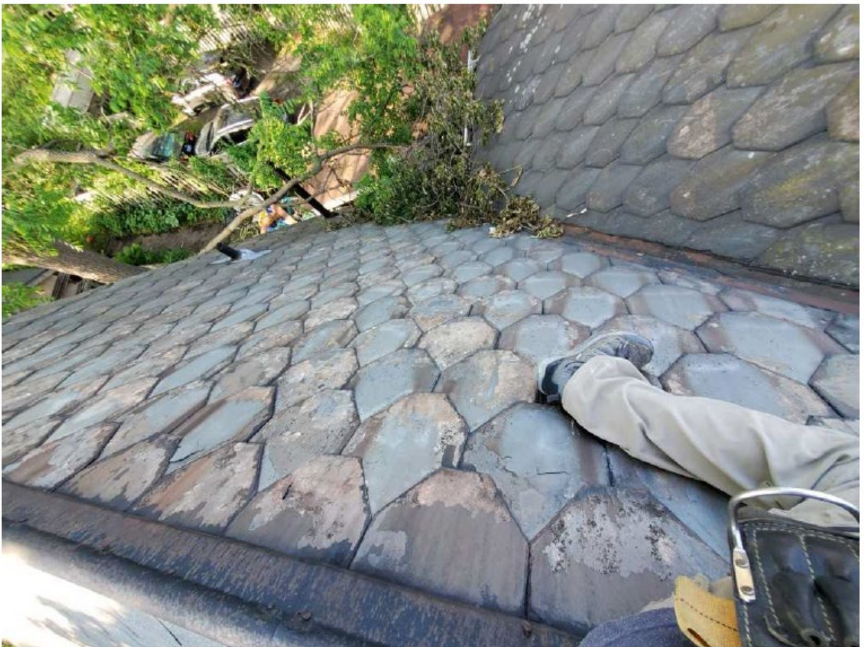
Image 14: Photograph submitted as a part of an inspection report showing extent of damage to the slate roof.
