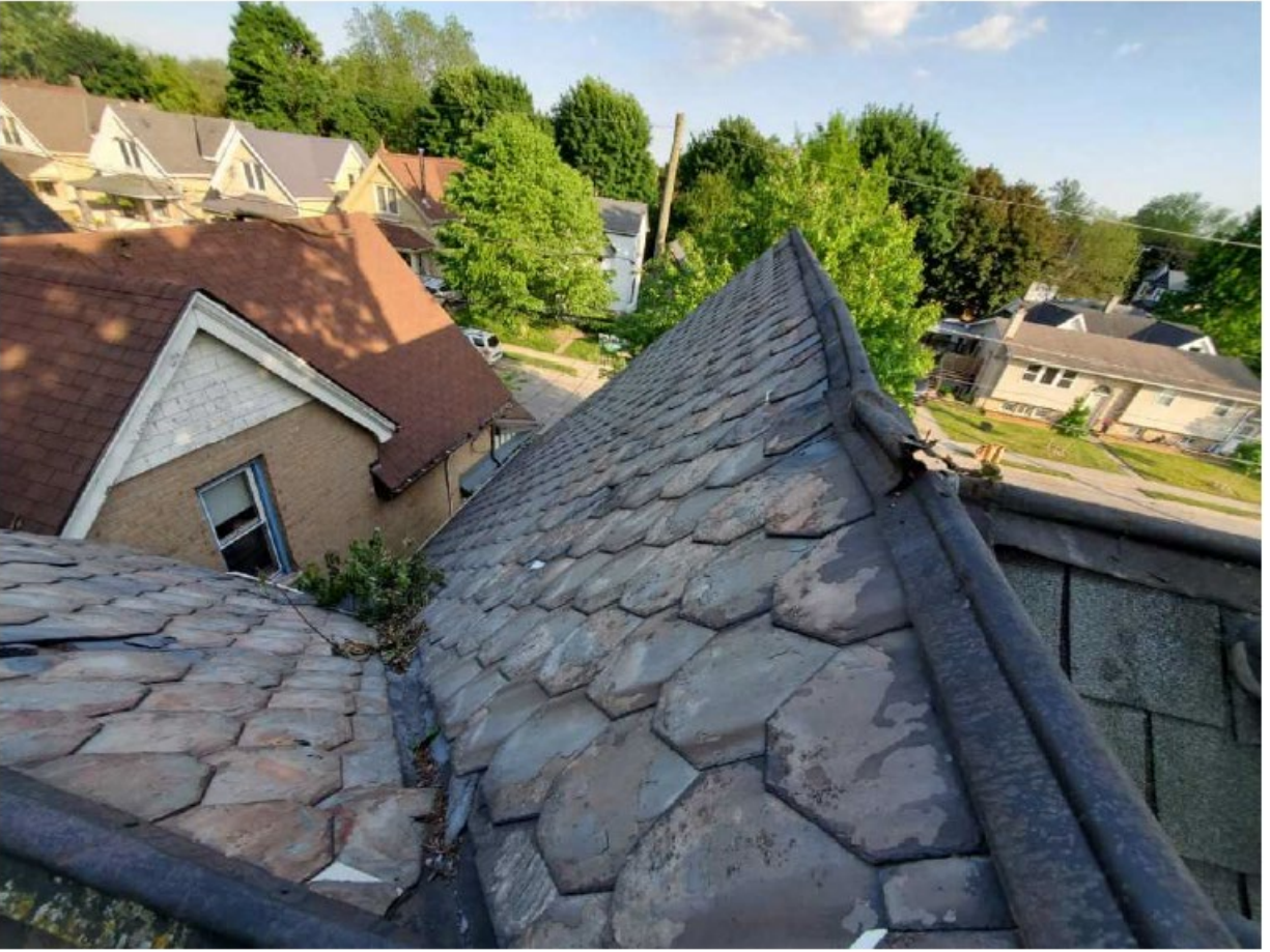
Image 12: Photograph submitted as a part of an inspection report showing extent of damage to the slate roof.
