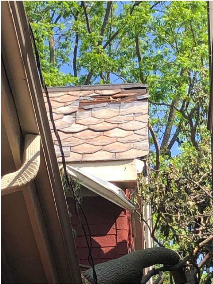
Image 7: Photograph submitted as a part of an inspection report showing extent of damage to the slate roof.
