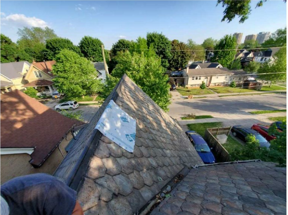
Image 9: Photograph submitted as a part of an inspection report showing extent of damage to the slate roof.
