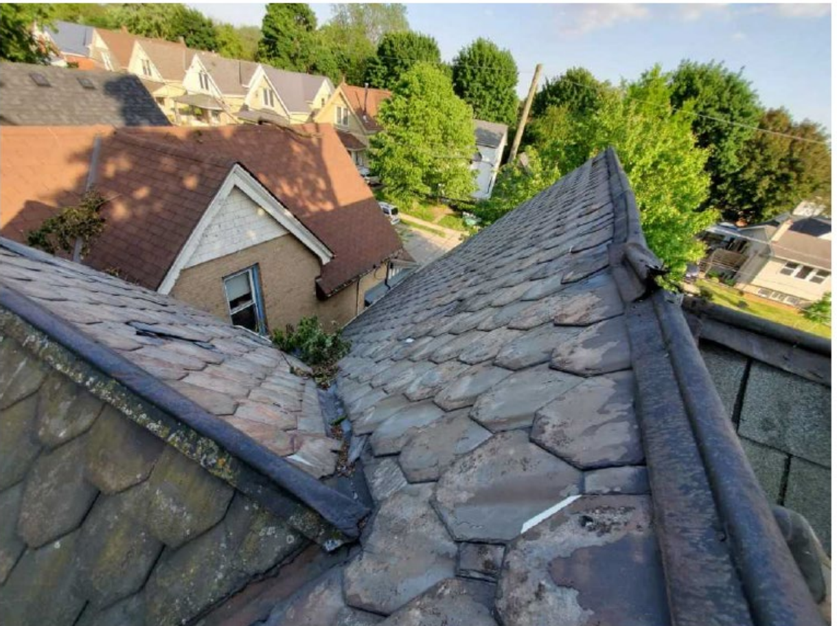
Image 10: Photograph submitted as a part of an inspection report showing extent of damage to the slate roof.
