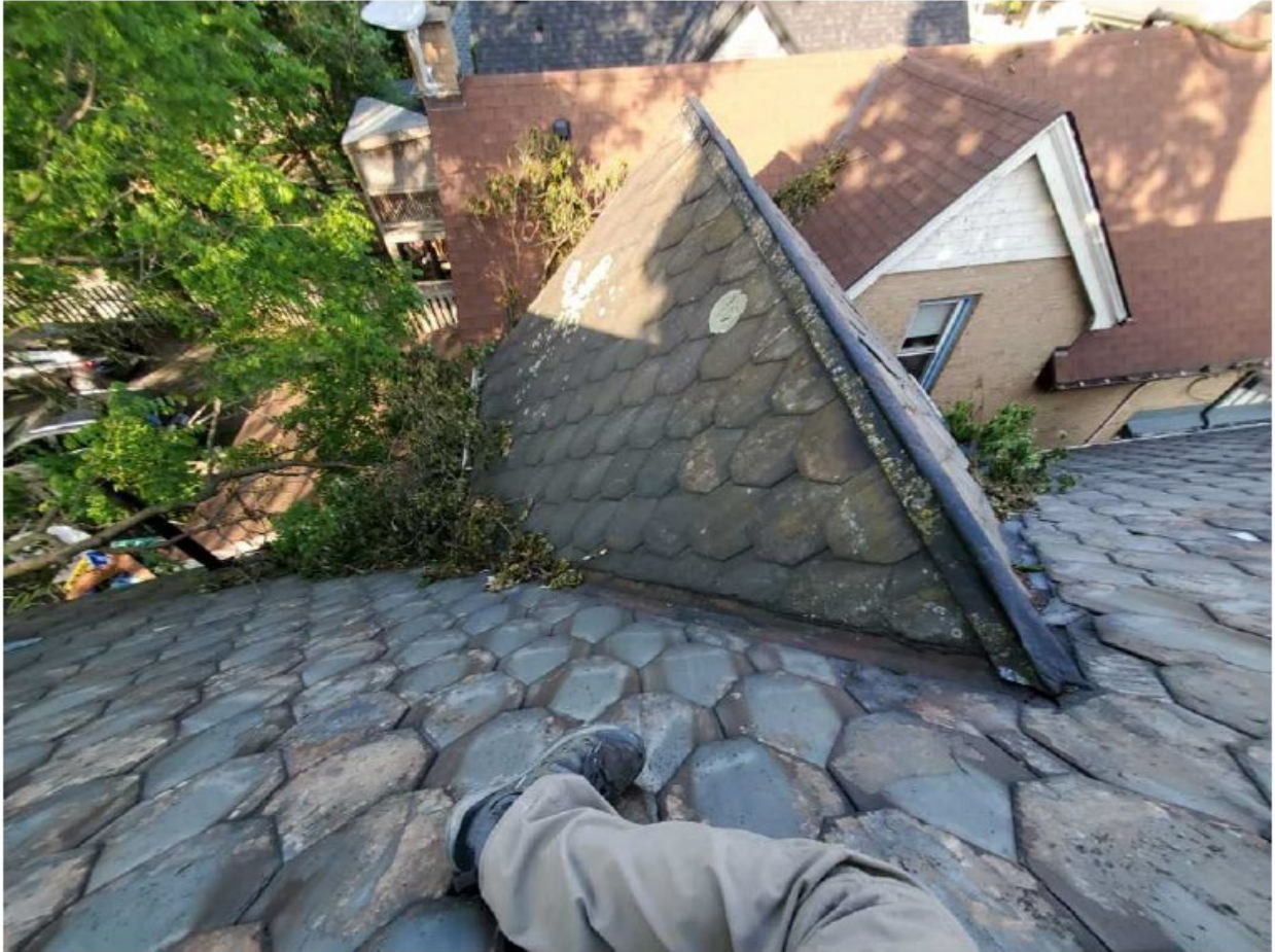
Image 13: Photograph submitted as a part of an inspection report showing extent of damage to the slate roof.
